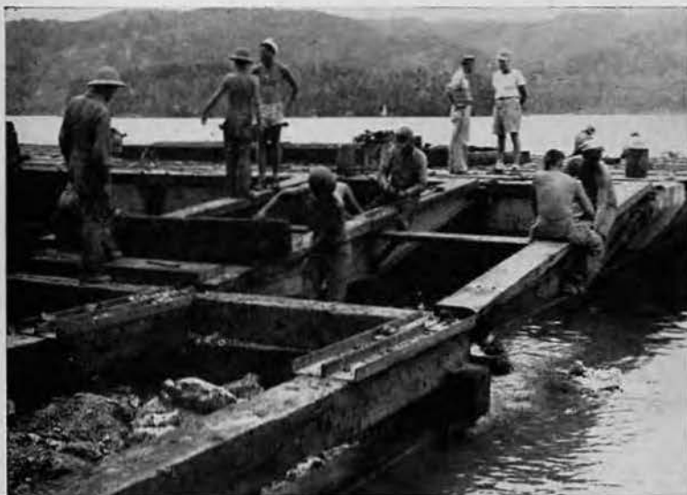
THE DETAIL. Heavy ramps from pier to shore are put into place. Timbers for the ramps were made of heavy native lumber cut to order by battalion sawmill. Four ramps of this type connected the pontoon pier to the land. Such work had to be right.
