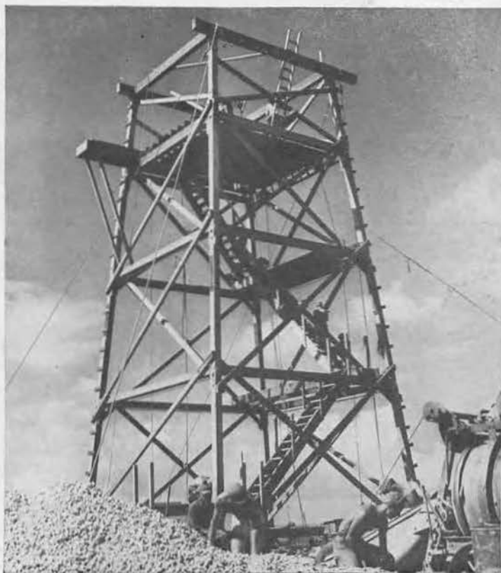
TIE HER DOWN! As framework nears completion, stairs are installed and deck for radio generators built. Cement gang shovels mix into hopper for concrete base that will help anchor tower when Okinawa typhoons come in September and October.
