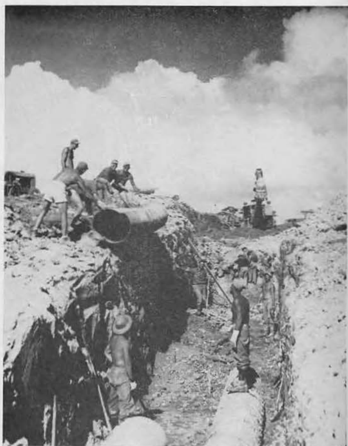
HEADS UP! "The Muck Gang" lowers another drainage section into the completed cat excavation. When the galvanized section reaches bottom, Chief Rychlak will order "all hands below" to move pipe a little to the port or a trifle starboard.
