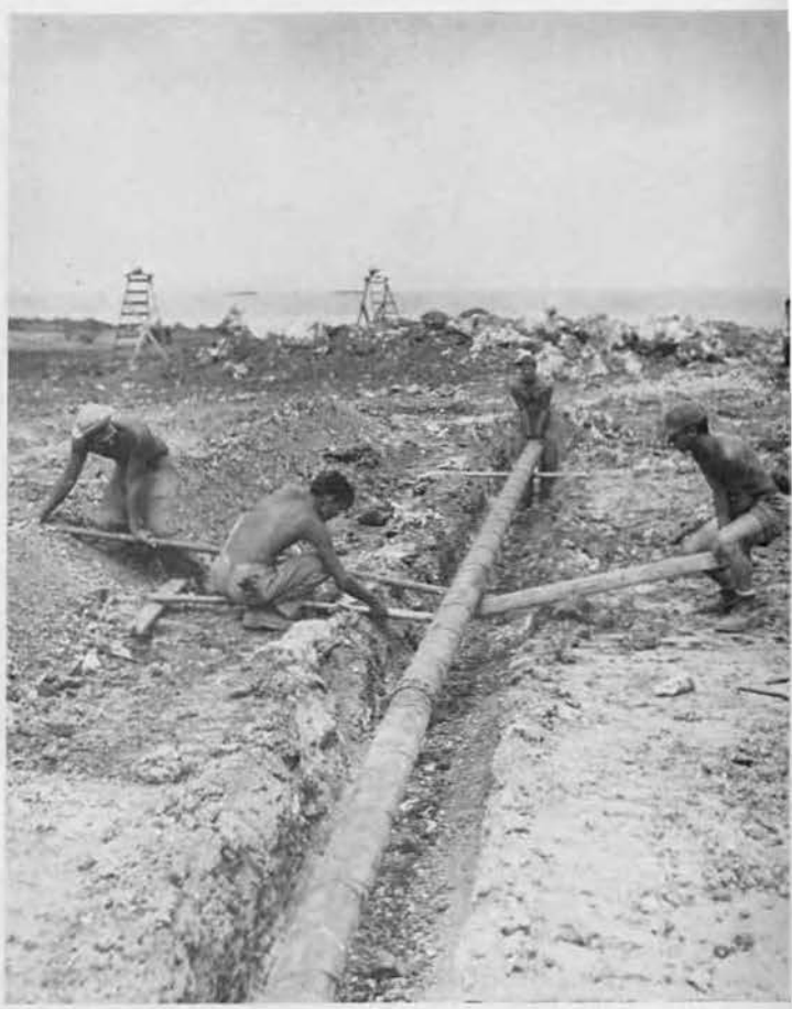
PINCHHITTERS. A carpenter crew is detailed to work at a common labor job—sinking one of four power and communications conduits running under the strip. Left to right: A. Thompson, Lowell Cable, Angelo Insalaco and William Beard.
