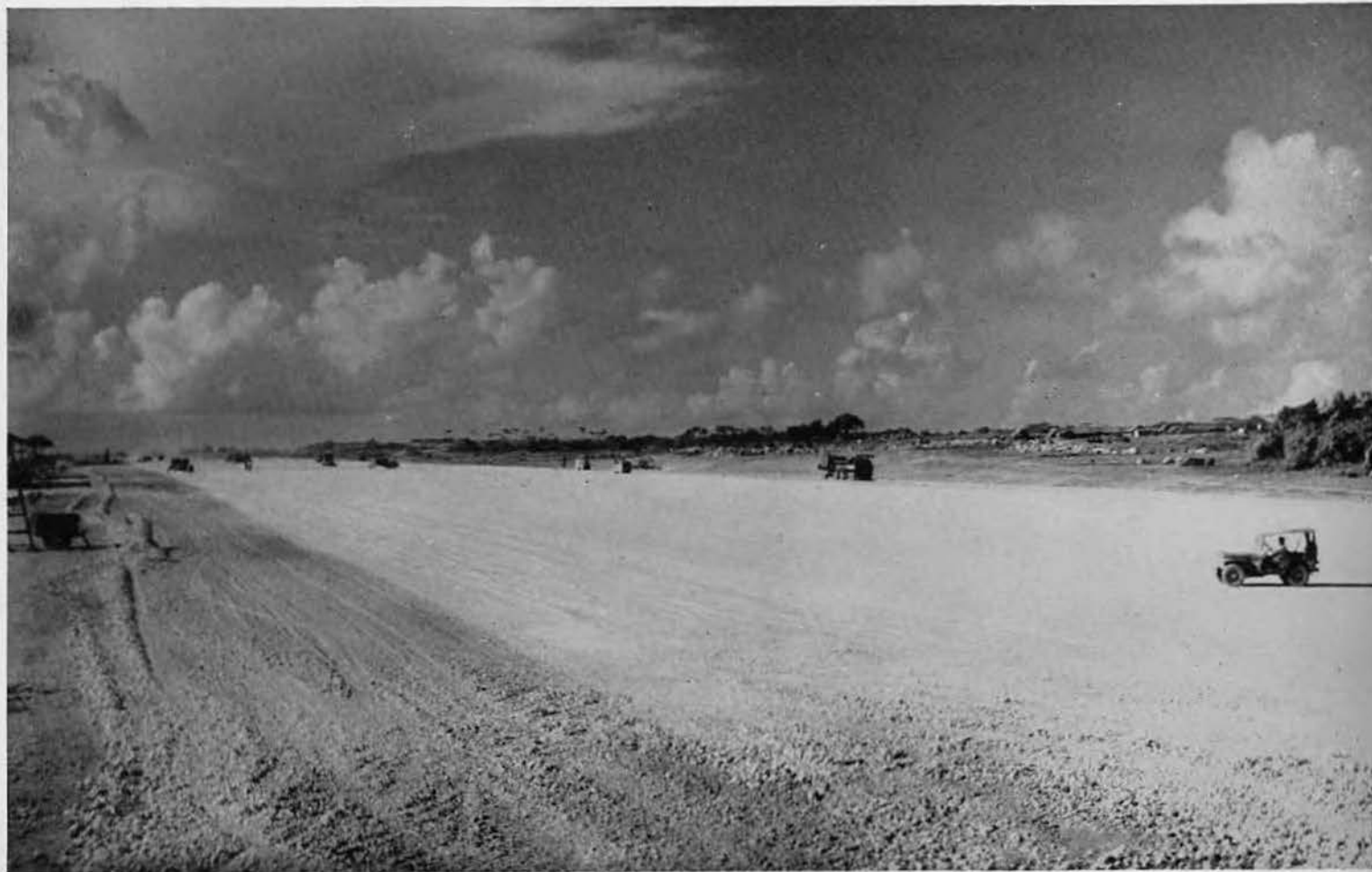
WELL DONE, BOYS! Comdr. Cook (in jeep at right) gives completed south end of Bolo runway the once over as only an experienced construction veteran could do. It was indeed a rare day in June (or July) when THE MAN didn't visit his favorite project now that Yontan was no longer
