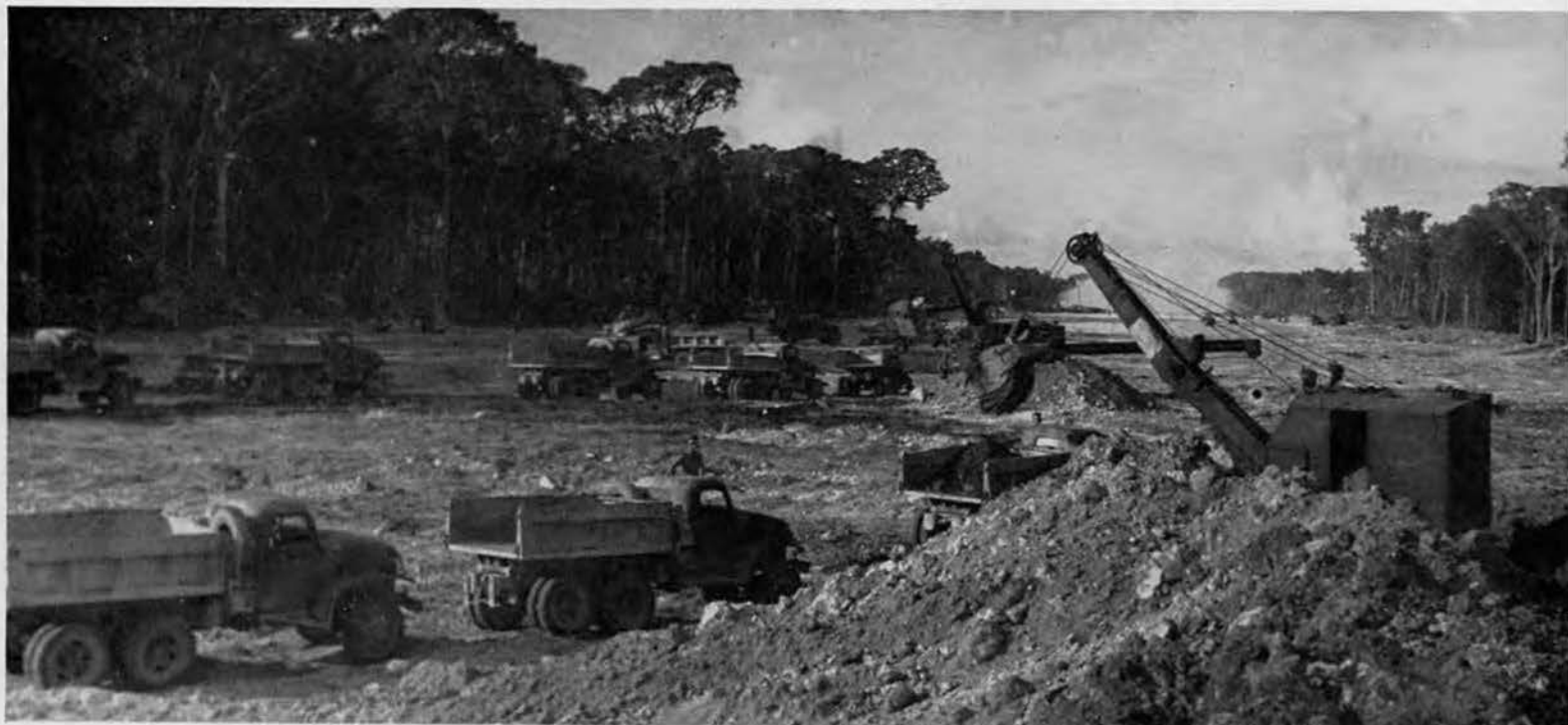
EARTHMOVERS EXTRAORDINARY. In foreground, bulldozers have pushed waste humus material into large piles from which three-quarter shovels are loading trucks. Further back (left), pans are engaged in final stripping. A group of pans (background) are cutting and filling coral, bringing the
