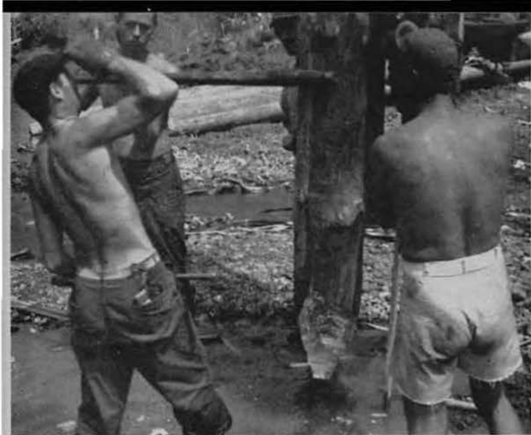
SIX O'CLOCK SIGHT PICTURE. Sloshing in rivers and muddy streams, the 87th pile-driving crew was soaked to the skin from morning to night. Paced by big "Spook" Elliott (left), the gang included: Warner, Hewitt, Hoback and Rooney.
