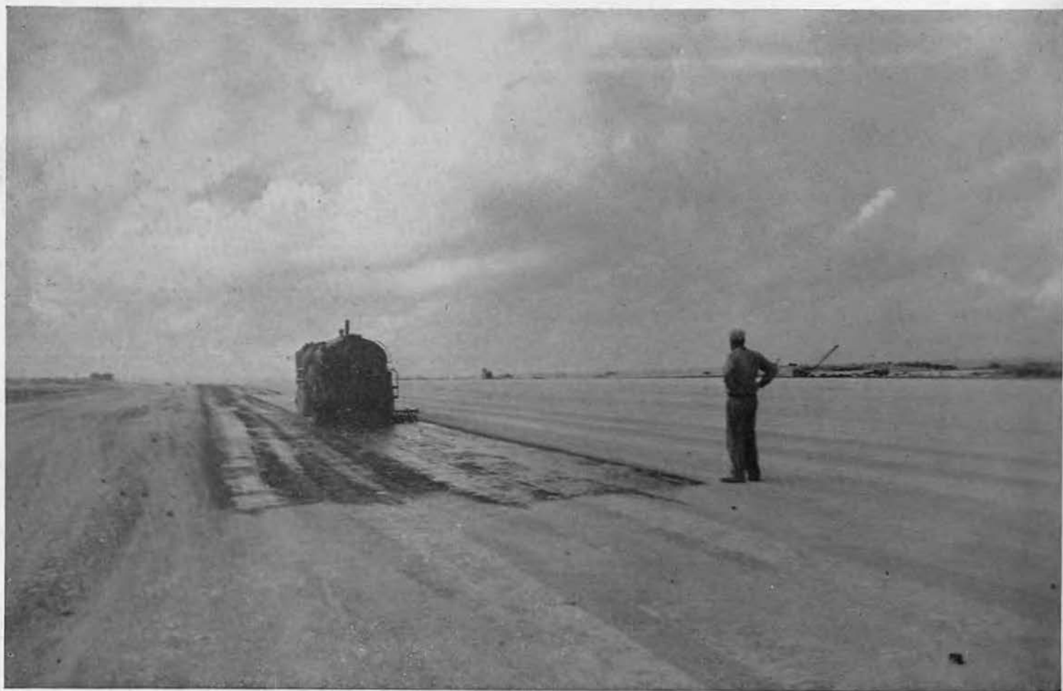
FINAL APPLICATION. Black-topping of the completed Bolo runway is started at northeast section of the strip. Towed by a 10-wheel truck, trailer tank has a sprinkler attachment that spreads a 10-foot section at a single
