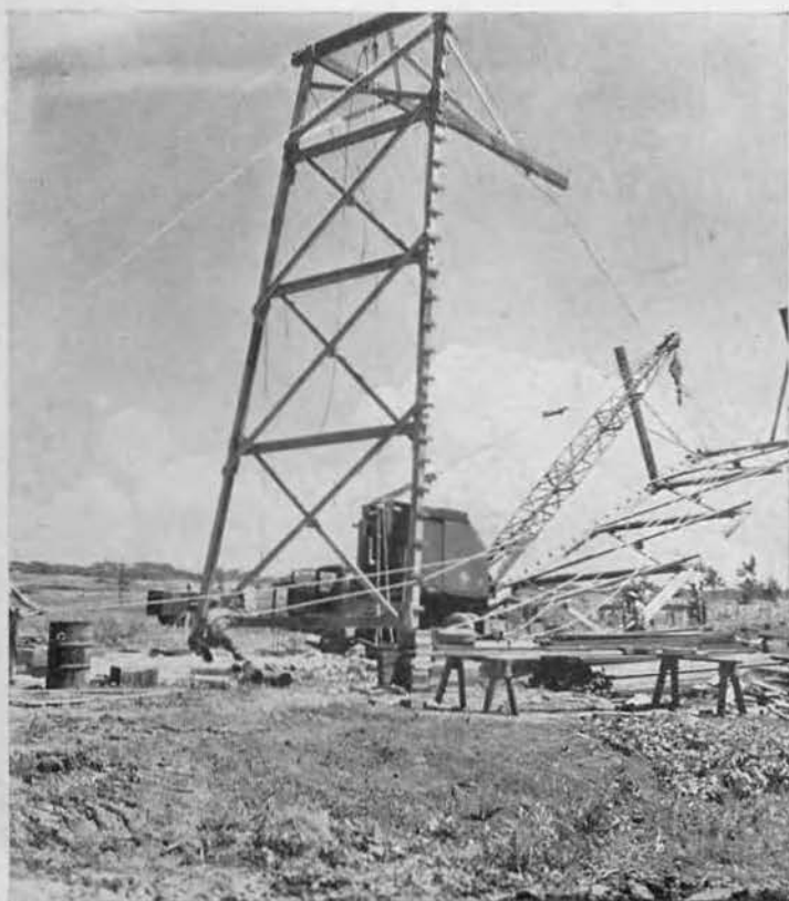
GOING UP. Bolo control tower finally begins to take shape despite the AAF changing its plans four times after construction had started. With one section in place, a crane lifts the other side and soon the sections will be tied together.
