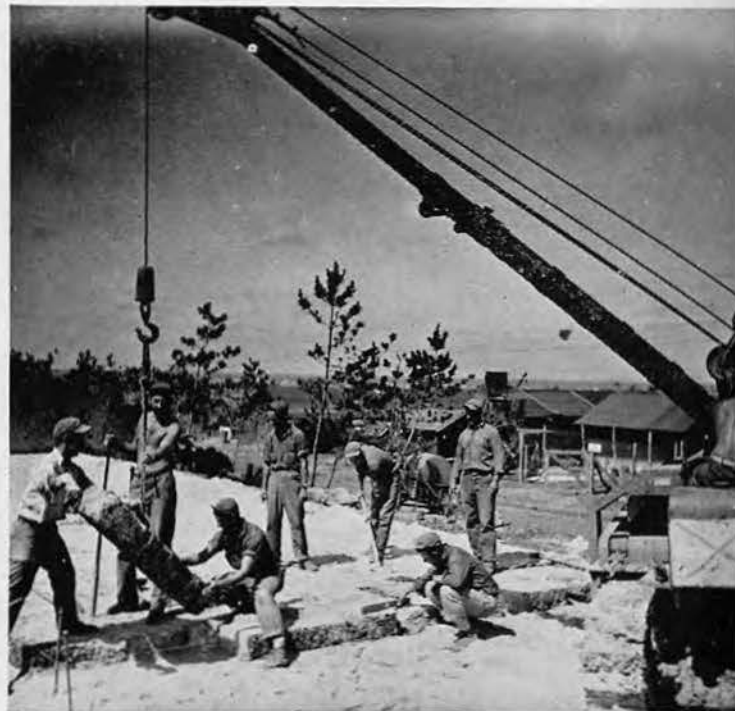
ROBBING THE OCEAN for these "just right" coral blocks cut by natives from conveniently located reefs, Chief Doug Thomas (standing, right) and his versatile concrete gang lay foundations for Ship's Store in May. Chow hall is in the background.
