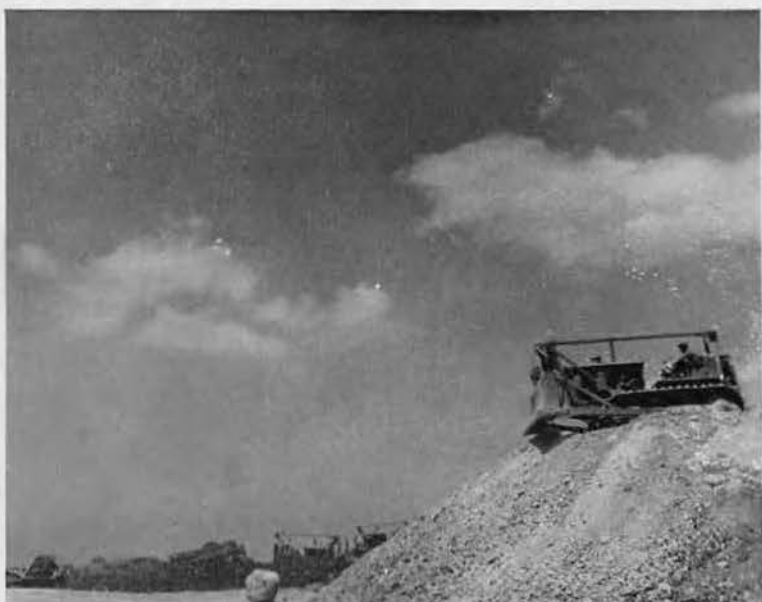
TRIMMING deep fill slope at western end of lengthened, reinforced Jap strip, one of many 'dozers pushes another load over the side. This temporary measure kept badly needed field from being closed to all planes. Pans (center) grade new location.
