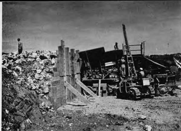
FIRST UNIT of the rock crusher assembly at Nagahama Quarry is being erected as the jaw crusher is set in place. Heavy timber bulkhead, set against formidable earth ramp (left), provides an easy approach for rock-laden trucks.
