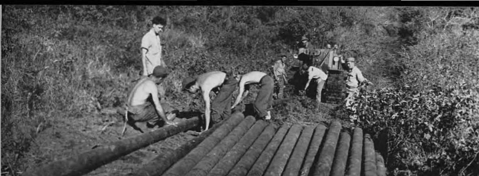
WATER MAIN. Laying the principal waterline into the Monte D'Or camp involved skinning the heavy pipe a distance of approximately two miles over the rolling, scrubby hills adjacent the towering mountain range. An
