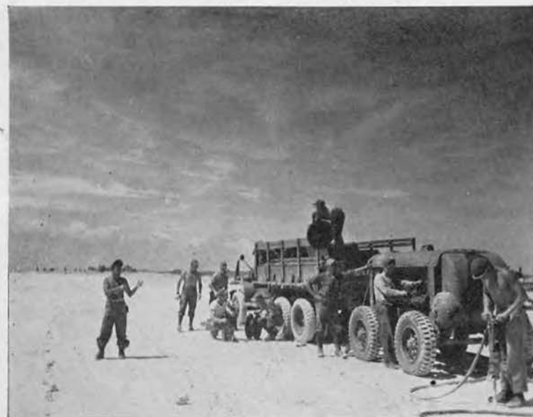
DYNAMITE CREW removes coral chunks from the graded pavement. Those present: Manuel Rivera, Dick Henry, Harry Jolley, Bill Listenberger (kneeling), Clarence Keller, Paul Armstrong (on truck), Chief Al Broomfield, Leo Burke and Jimmy Beachler.
