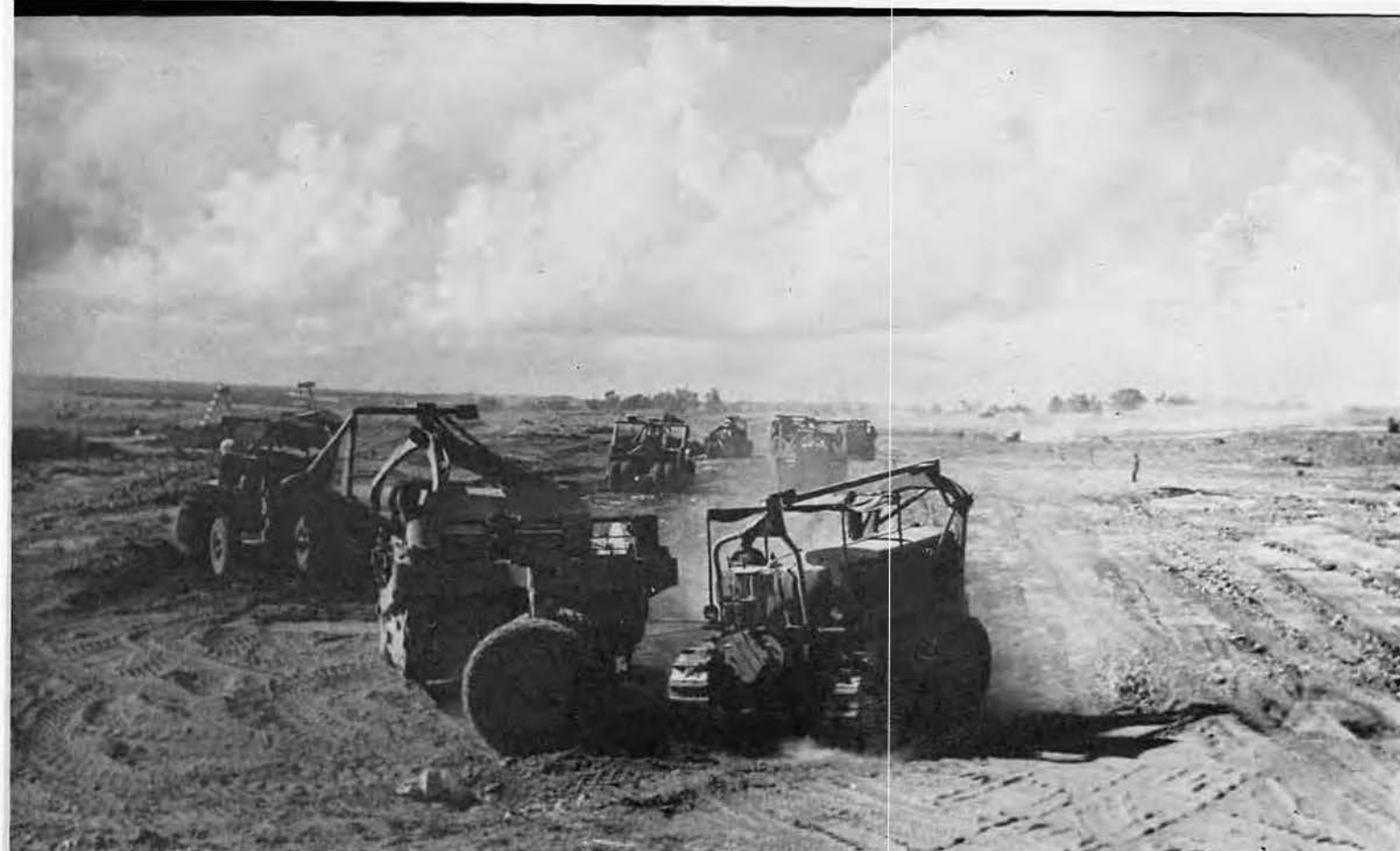
30 DAYS ALLOTTED. Perfect weather for large scale earthmoving prevailed during virtually all of the 30 days allotted for the construction of Bolo's first B-29 strip. The second of the twin strips was started, but cancelled by war's sudden end in August. Here, sub-
