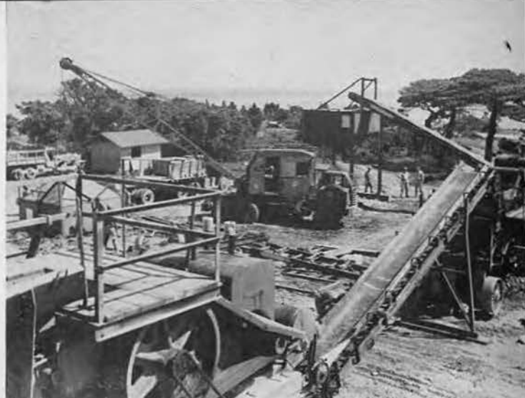
JIG SAW. Before the 87th could complete the assembling and erection of the new crusher, it fell heir to the full operation of the project. Soon the versatile Earthmovers were shooting down whole mountainsides (see previous page).
