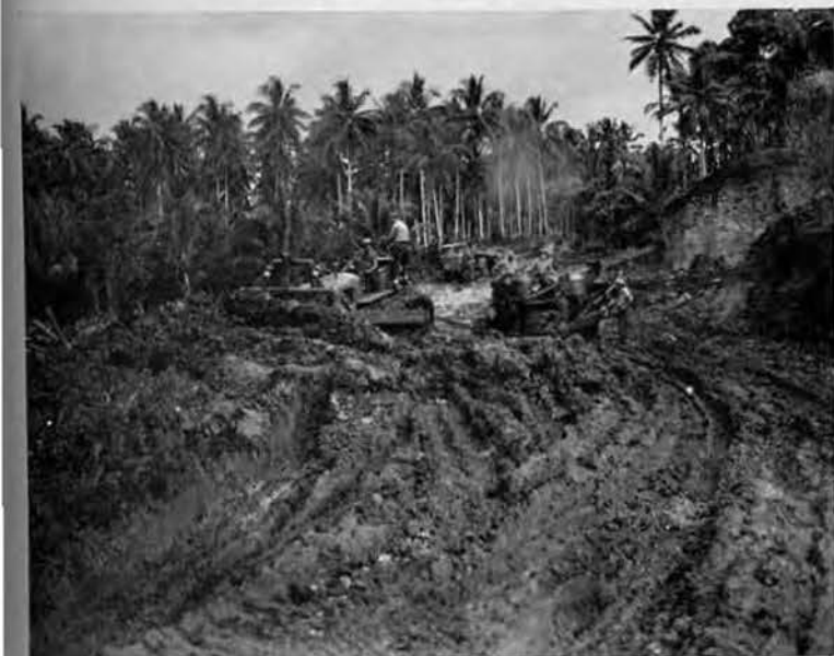
MUD. Even giant bulldozers sometimes bog down in tropical mire. Here, Tom Hutson rescues "Chet" Wlostoski and his stuck 'dozer from the muck. Huge fills in swamp made this road project a stiff proving ground for both men and equipment.
