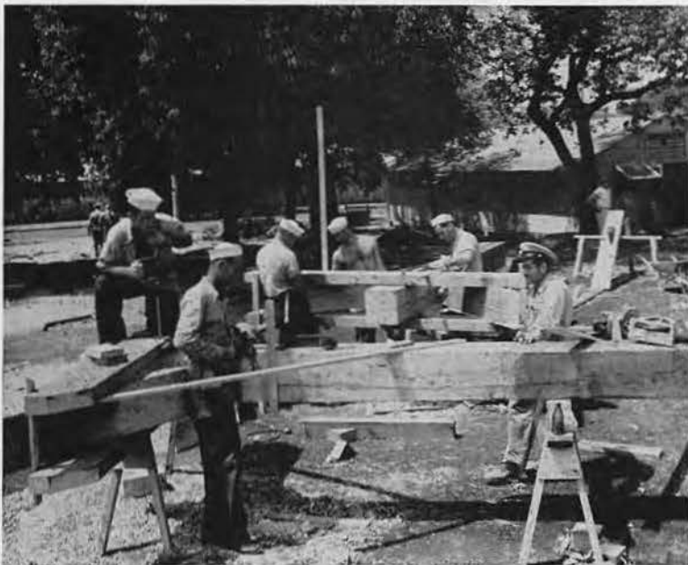
ACROSS THE STREET from thriving TRADE WINDS (see picket fence), Chief Rufus Bland (right) directs construction of foundation for projection booth. Carpenters are: Darrell Haws, Julius Scruggs, Joe Williams, Daniel Petrich and Bob Droege.
