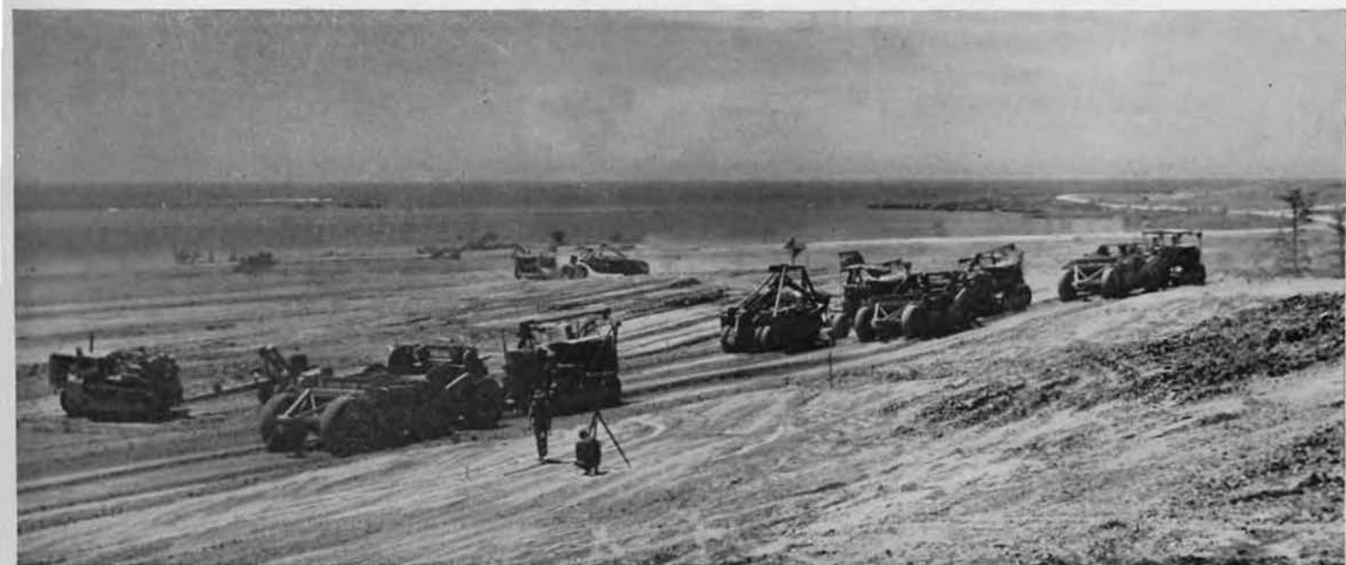
CARVINGS. The sloping hillside at northern end of Bolo runway is being carved away by a battery of pans. Earth from this cutting operation is being hauled leftward to fill in connecting ramp with westerly taxiway. Eventually, this entire hill had to be cut through to connect with east
