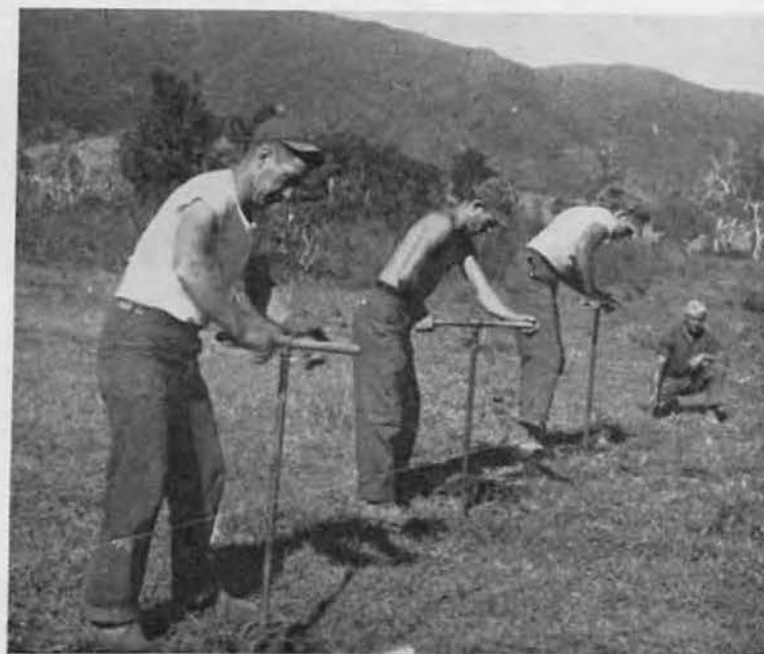
HEAVE HO! Miles of fence had to be reset by hand to make room for the road widening. Chief Al Broomfield (right) directs a straight line for the post-hole diggers, who are (left to right): Listenberger, Perlak and Ahlf.
