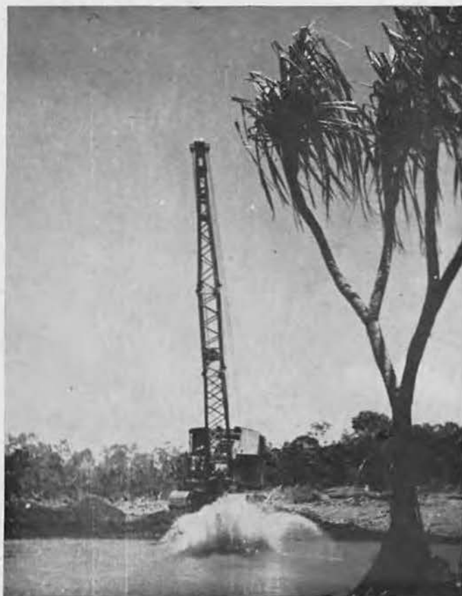
SPLASH. Final gravel-topping for completed stretches of new road was scooped out of handy stream bottoms with the dragline. Splash resulting from this operation was fodder for visiting picture book cameraman. Semi-tropical tree adds class to shot.
