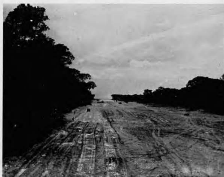
PROGRESS. The dense Solomons jungle stubbornly yields to the furious onslaught of the Seabees. Things are looking better as the Strip begins to take shape. In foreground (left), a 'dozer prepares site for a twin .50-mm. ack-ack gun.
