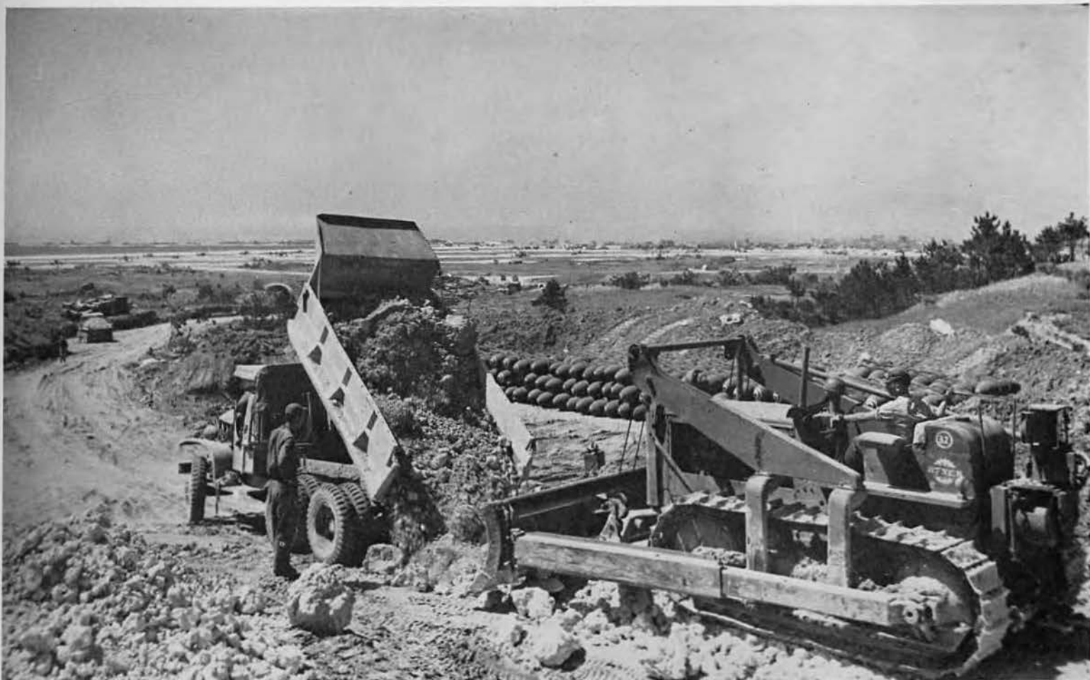
IN THE DUMPS. "Kask" Conine dumps a load of rough coral on newly constructed access road into Yontan bomb dump as Meredith Walls (standing, left) checks grade. Oliver Aulry (right) operates the 'dozer. A pile of 500-pound aerial bombs stacked in the revetment may be seen, in part,
