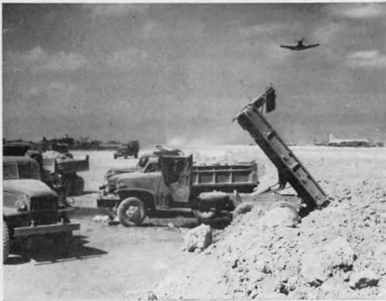
LOAD AFTER LOAD of coral is dumped at edge of runway by some of 87th's 30 trucks employed on battalion's first Okinawa assignment. One of hundreds of Corsair fighters of the Marine Air Wing operating from Yontan flies over.
