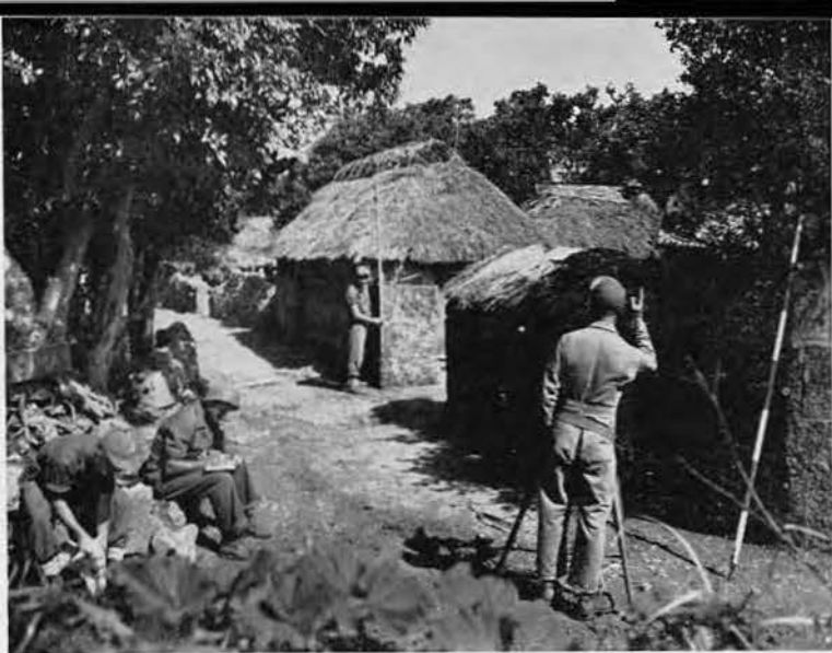
PRELIMINARY survey for Bolo Field, which ran through village of Jima, was 1,700 feet east of site where B-29 strip was finally built. Members of Chief Paul Sowers' (left) survey gang shown are: Sam Fields, August Kafer, John Barker.
