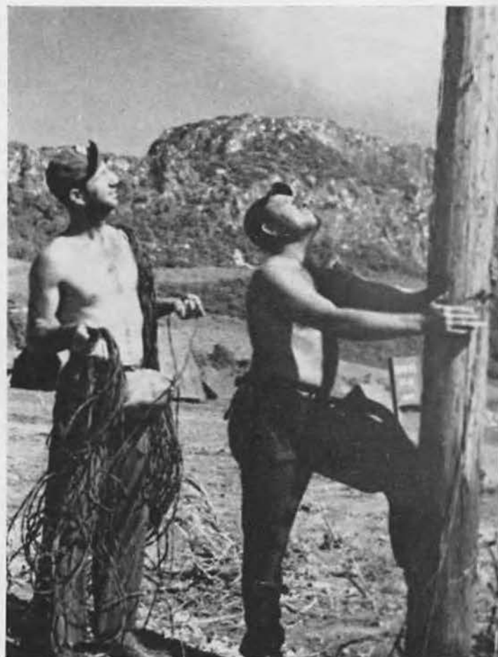
WIRED FOR ACTION. William Shady (left) "gets a line" on pole as Andrew ("Mule") Steadley prepares to mount native timber. Altogether, 50 miles of telephone and 20 miles of electrical wire knitted the staging camp into a tightly-woven unit.
