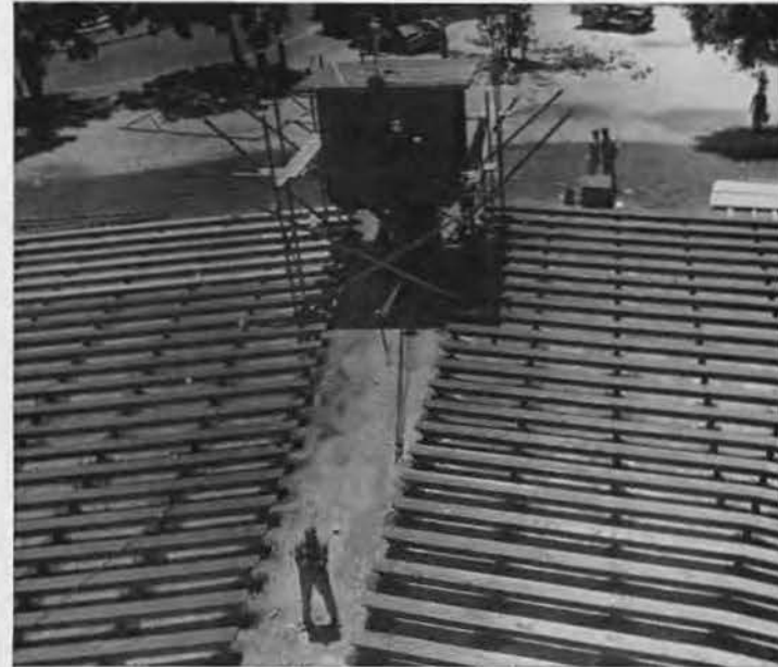
PROJECTION booth almost finished and seating arrangements for an audience of 1,200 ready. Chief William Martin (arms folded) focuses attention on few remaining touches needed to complete stage. EARTH-MOVER photographer found theatre an arresting subject.
