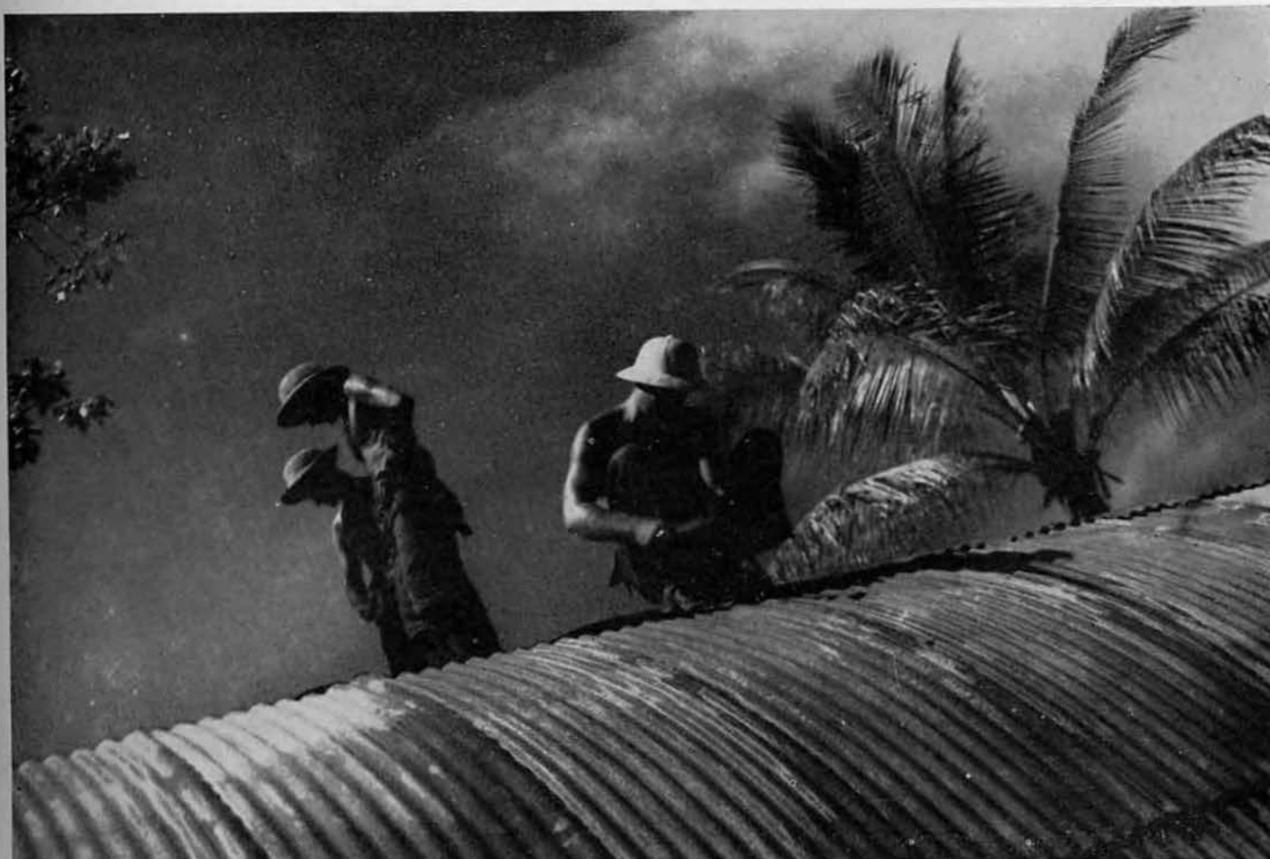
TOPPING IT OFF. Richard Bogdanski and Charley Danford consult on the finished product while Clarence Nielson nails last section of quonset roof in place. While working in the open, sun helmets were a necessary item of apparel. Tender, young palm at right (one of a few growing any dis-
