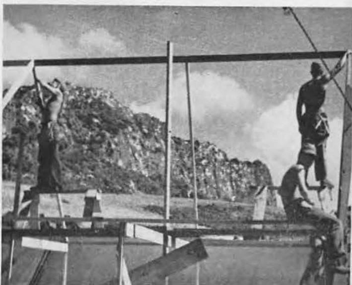
FRAMED. Warren Parrish, Joe Ward and unidentified carpenter's mate are shown in midst of framing battalion barber shop, which will be ready for customers once a tarp covering is thrown over skeleton. All staging structures were strictly temporary.
