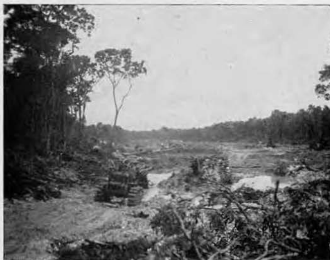
HITCH-HIKERS. A "snatch-cat" tows a huge stump and carries a couple of passengers. The small tractors had been used previously to drag logs out of the rough and up to the loading pits. It has been raining again!
