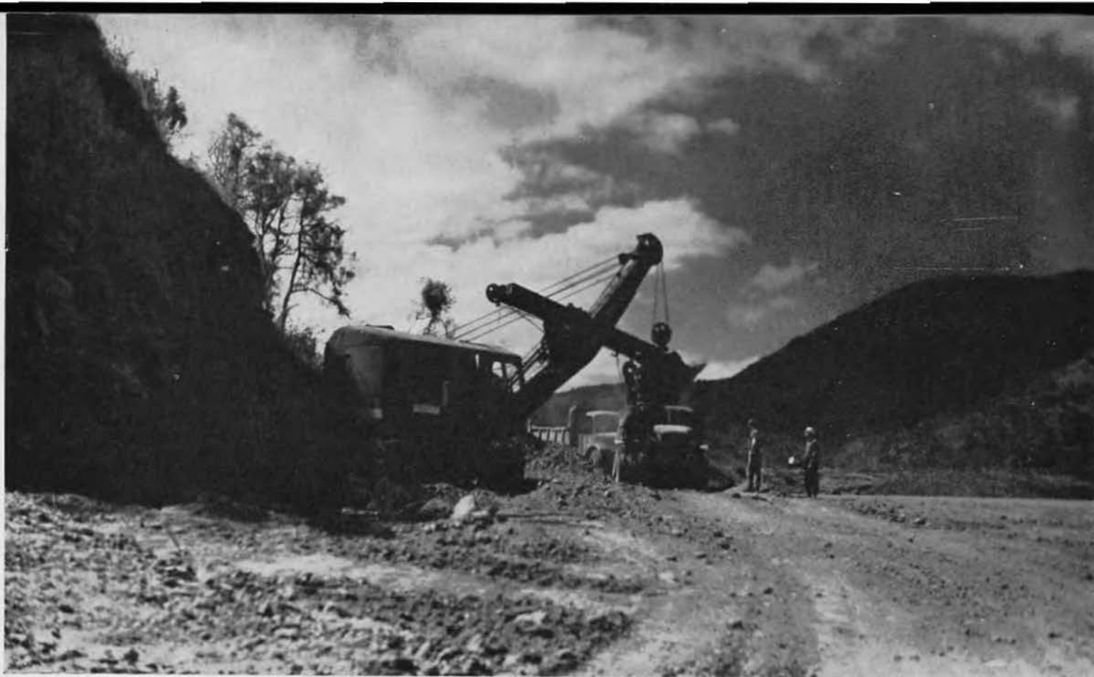
FACE LIFTING. The big Northwest shovel was kept busy tearing out huge chunks of the mountainside, which bordered the road project. Transporting the above monster and other heavy equipment the 133 miles between Monte D'Or and the Bourail location presented a major traffic problem.
