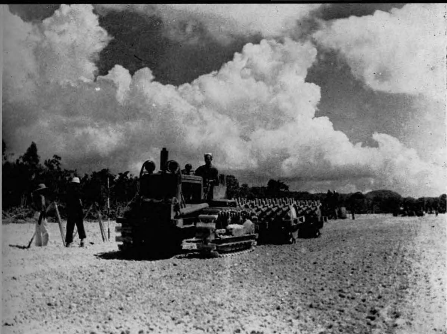
WALKING OUT. All fills were considered properly compacted when the sheepfoot roller "walked out." The sheepfoot also proved itself invaluable with its ability to spread large chunks of soft coral into smaller ones, thereby speeding up the operations immeasurably. Here, R. F. Johns is operating the sheepfoot rig. Surveyors Tom Campagna and Byron Chronic (with transit and levels) are setting blue tops. Grade Foreman Jim Bailey, (staff in hand, right) is supervising operations. Grader operator is C. J. Rominger.
