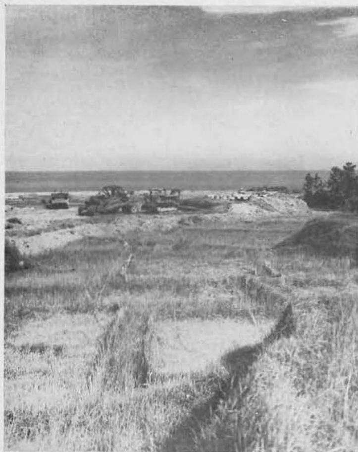
RICE PADDY. This obstacle, harmless in appearance, but a formidable obstruction to rapid construction, had to be drained before strip could cross over. A 12-yard pan is doing preliminary cutting on culvert ditch before backhoe takes over.
