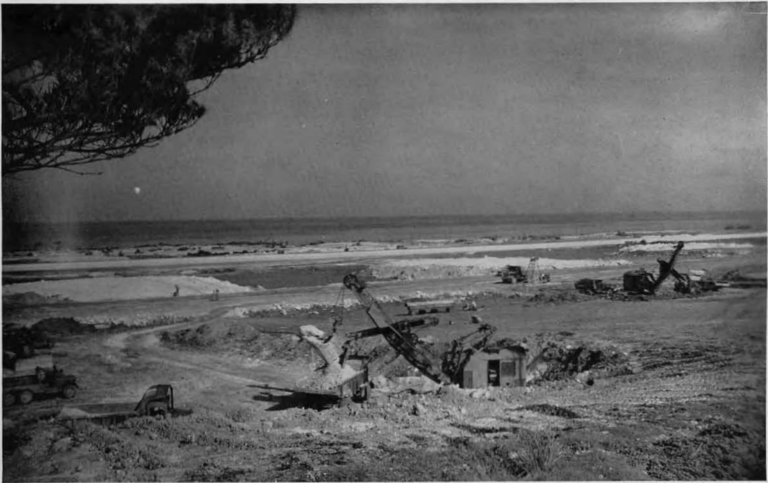
LOOKING WEST across Bolo Field to the East China Sea, a 2½-yard shovel loads a Euclid with one of last loads of coral used. A 1½-yard shovel (right) digs dirt out of last hardstand. In 1943-44, Stirling Airfield
