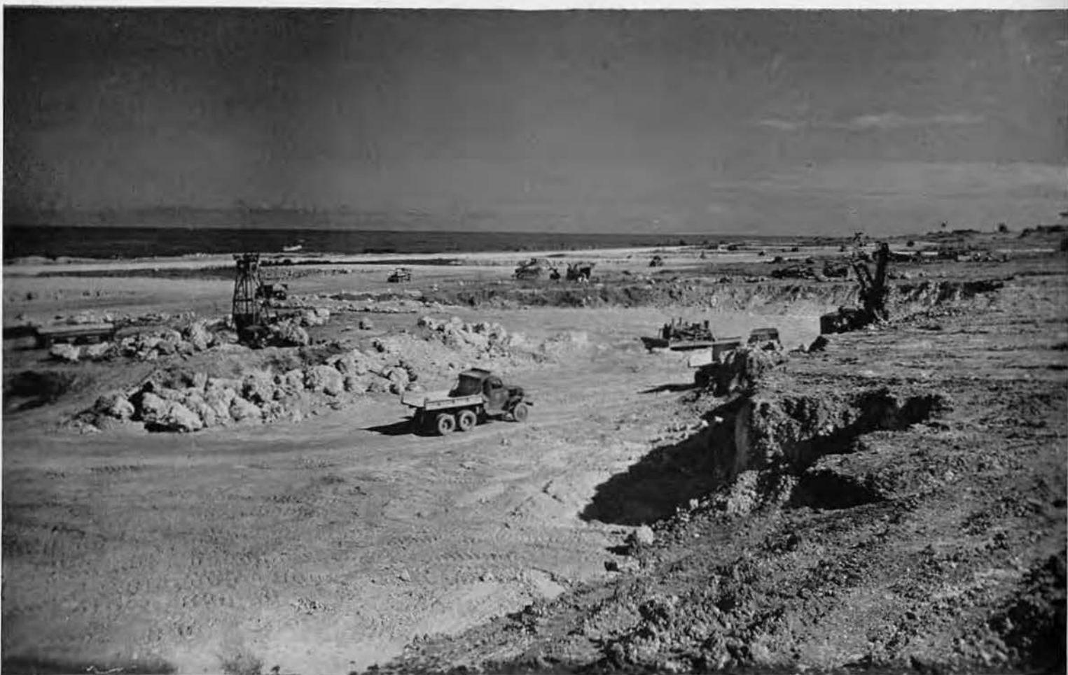
CUTTING ON "C" taxiway goes ahead as pans cut out adjoining hardstands on taxiway east of the completed runway. Most battalion equipment has been moved to this location. To the right of light tower are a few remaining piles of asphalt barrels. A roofer, pulled by 'dozer (right center), softens up the cut for pans. Tails of the new Douglas A-26 attack bombers (far right) are barely discernable. The taxiways at right are already completed and ready for occupancy.
