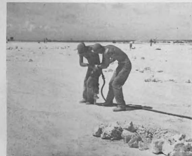
DIGGING FOR NUGGETS. A jackhammer crew is removing hard rocks from surface of runway. These "niggerheads" cropped up during blading and had to be dug out. The holes were then refilled with firm coral and the rocks thrown away.
