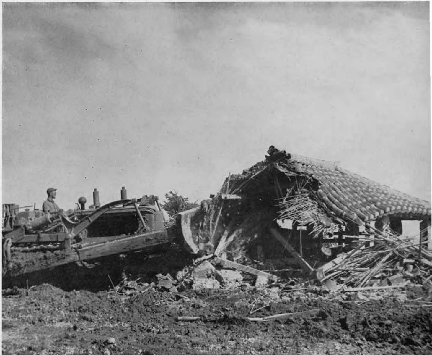
DESTRUCTION FOR CONSTRUCTION. This humble native home was directly in the path of an urgently needed road from the main highway to Camp Bolo. After battalion carpenters had salvaged all usable lumber (along with souvenirs and a colony of fleas!), "Big John" Wines
