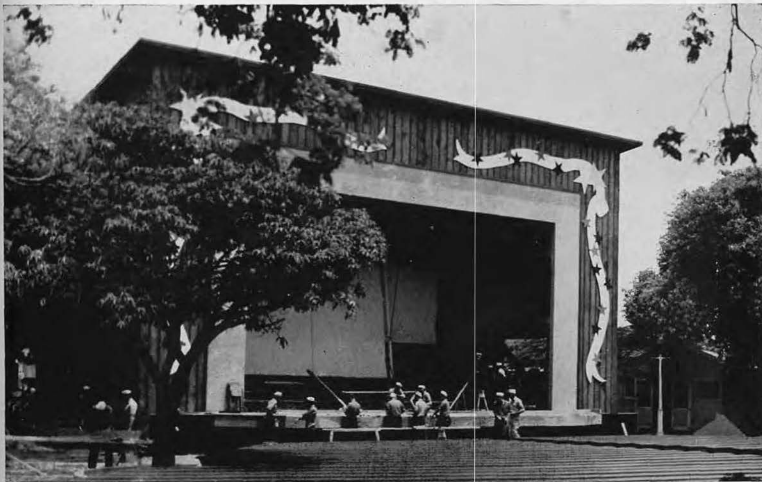
NOUMEA THEATRE. Finishing touches to new theatre were rushed to meet the deadline of 23 December for the colossal Red Cross Christmas Festival. Carpenter crews worked feverish 14-hour shifts and came to a breathless completion only four hours before the
