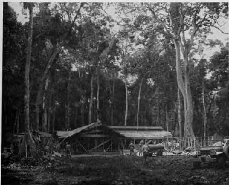
WHEN DO WE EAT? Eventually, the budding chow hall commences to shape up as skilled carpenters, assisted by muscular apprentices and laborers, hasten to complete the building so their shipmates might eat without undue exposure to the unpredictable tropical elements.
