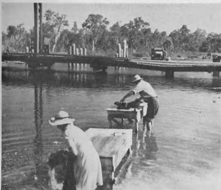
BLUE MONDAY. Every day was wash-day for the old French couple and their two attractive daughters near the bridge job. This frugal family had given up working the land in favor of the more lucrative hand-laundry business for Seabees.
