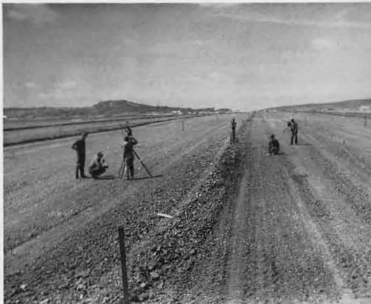
SUPER-RUNWAYS. "Plummy Rods" of 87th survey crew set up fill stakes on a section of sub-grade for paving. Big fills on old strip kept trucks busy continuously. Meanwhile, pans have shaped up entire length ready for coral. The airfield makers are clicking now.
