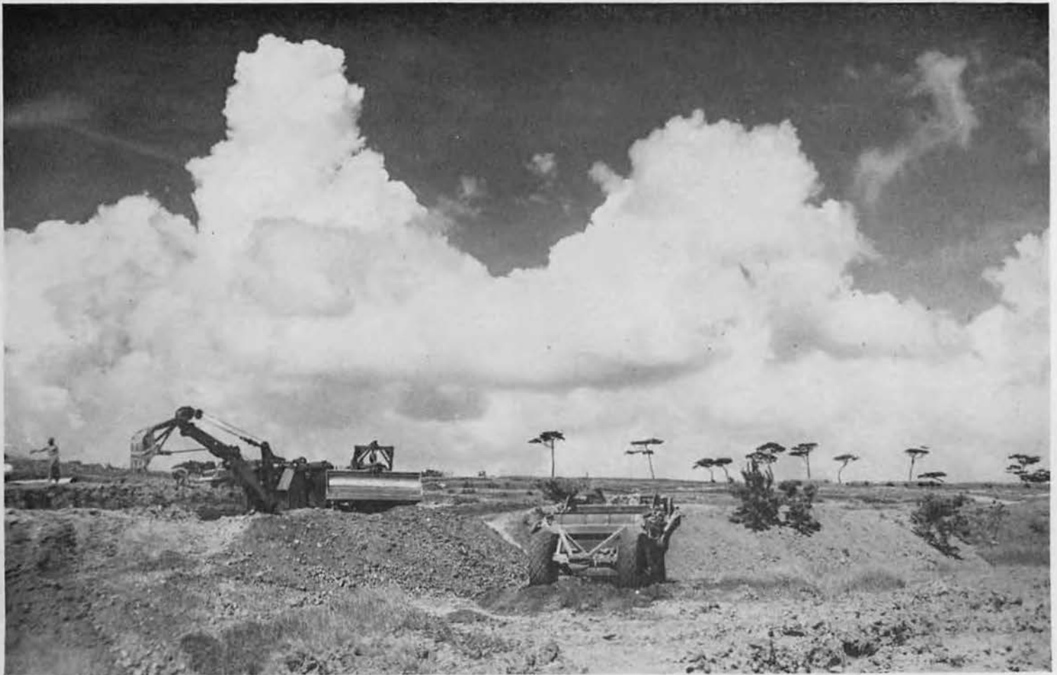
DIVERSION DITCH. The ditch that carried water away while metal drains were being installed is shown in right foreground. The pans have commenced filling in huge cut, which will be brought up to grade when culvert work has been completed. As fast as backhoe throws earth to one
