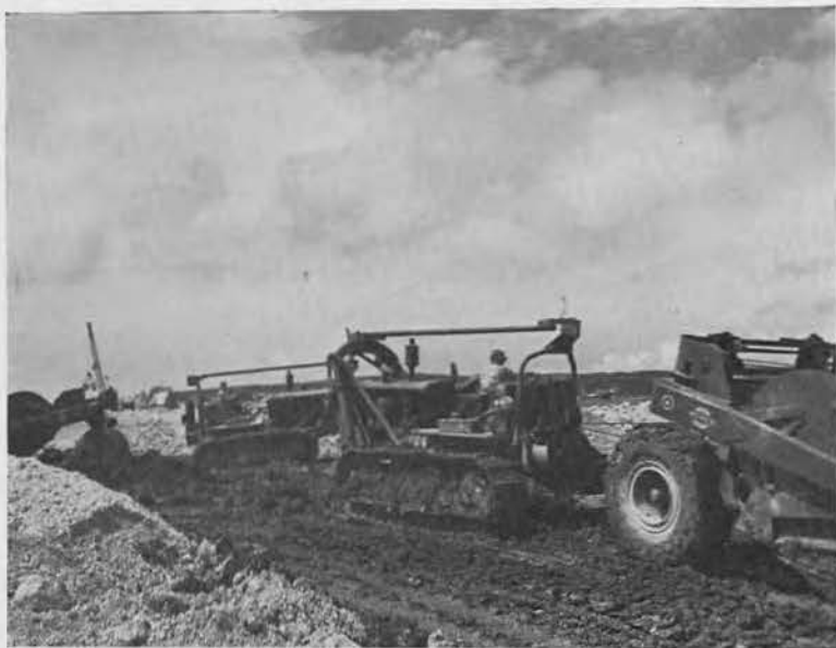
BAILING OUT the abundant mud from the sub-grade after the big rains was necessary before coralling could be resumed on Yontan Airfield. Ralph Carter (on dozer) pulls a pan at crossing of the East-West strip. Date: 15 May 1945.
