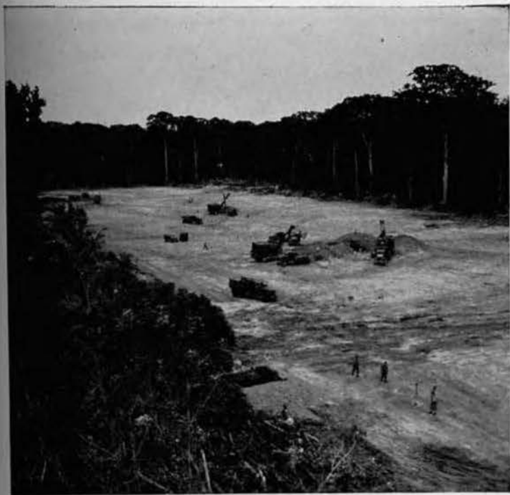
STRIPPING DOWN. This area is almost cleaned up. Soon the shovels can be moved to a borrow pit and the pan spread can come on through to perform its phase of the work. Excavations were former 90-mm. gun pits.
