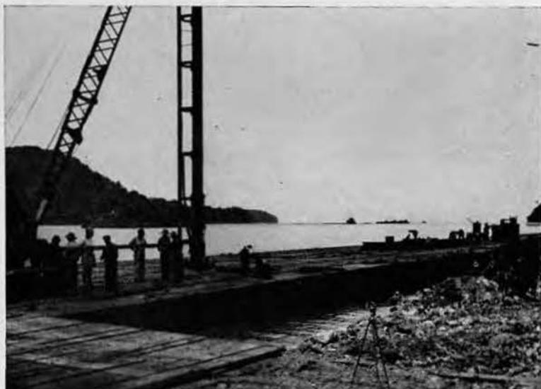
PILE-DRIVER rig is poised to sink one of many piles used for dolphins and clusters. Piles were sharpened and steel-tipped to secure them in coral bottom. Net tender and barge (right) are laying submarine net across harbor entrance.
