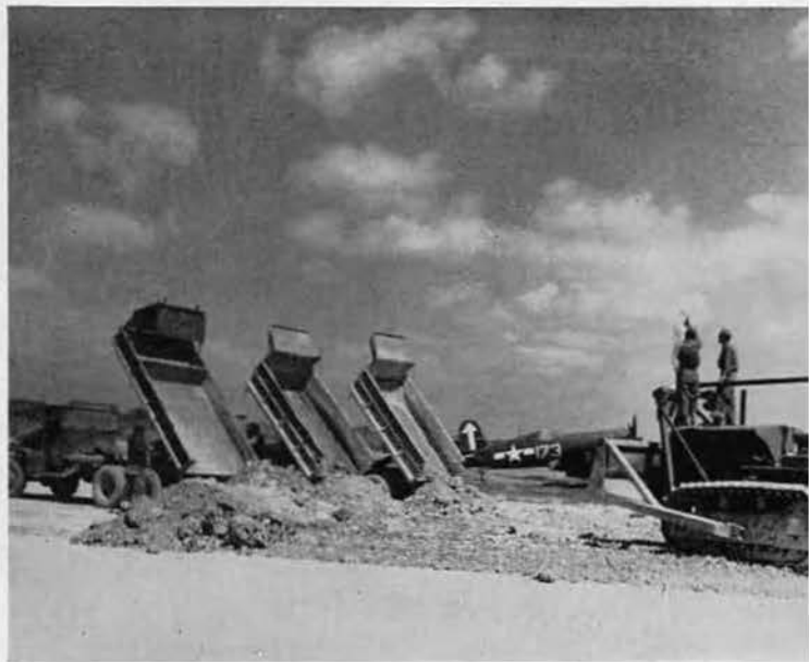
THREE OF A KIND are caught by alert EARTHMOVER cameraman as they dump additional paving material across old East-West Jap strip. Bulldozers will soon smooth piles to required level. A F4U night fighter is shown parked nearby.
