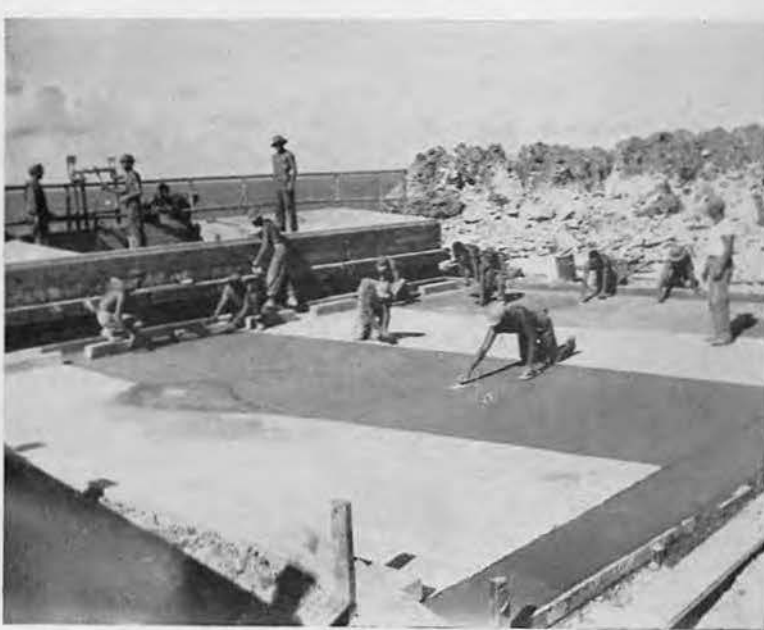
HONEST SWEAT gets a lot of fresh concrete troweled down to the right finish if you keep at it long and hard enough. Above, Chief Thomas' crew sweat it out on Bolo Point garbage disposal project. Here were some hard workers.
