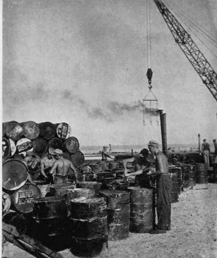
OPENING DAY. Using hammers and chisels, Seabees open endless drums of surfacing material. Thousands of drums were used as porous coral absorbed huge quantities of asphalt. A regular mixing plant was soon built at Nagahama.
