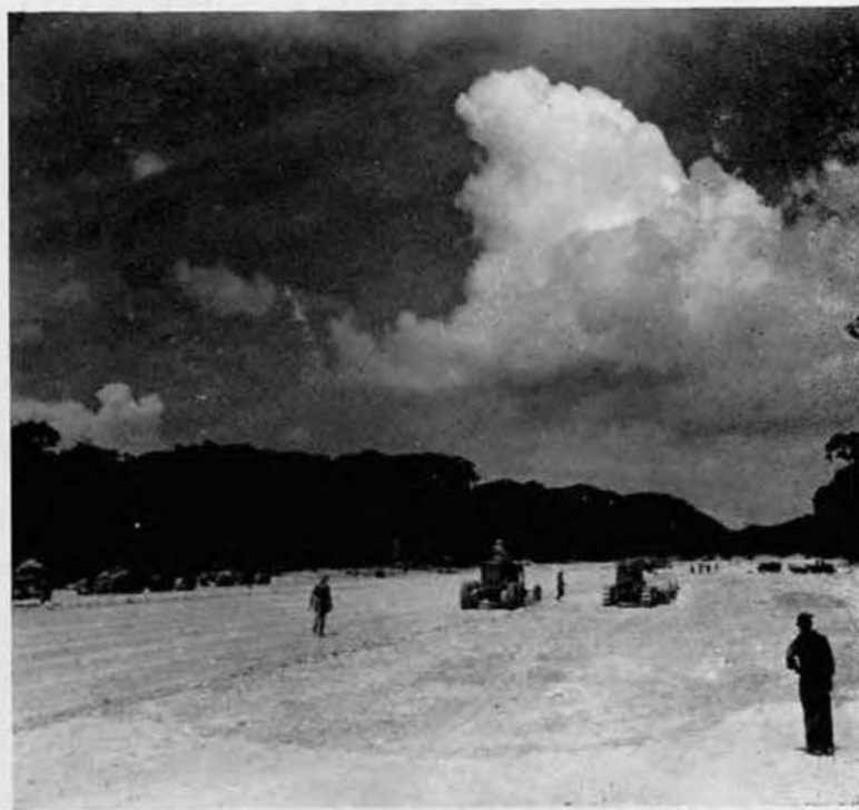
TAKING SHAPE. While pans are bringing the section to close rough grade (left), the grader is working the finish (right). Up ahead can be seen the demolition and donicker removal crew. (See page LXIII of CAN DO.)
