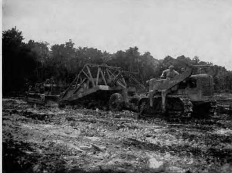
SKIMMING OFF THE MUD. Before grading the runway to shape, it was necessary to clear off the black humus overburden. Here, two HD-10s struggle to load an eight-yard pan with the sticky muck shortly after a terrific downpour.
