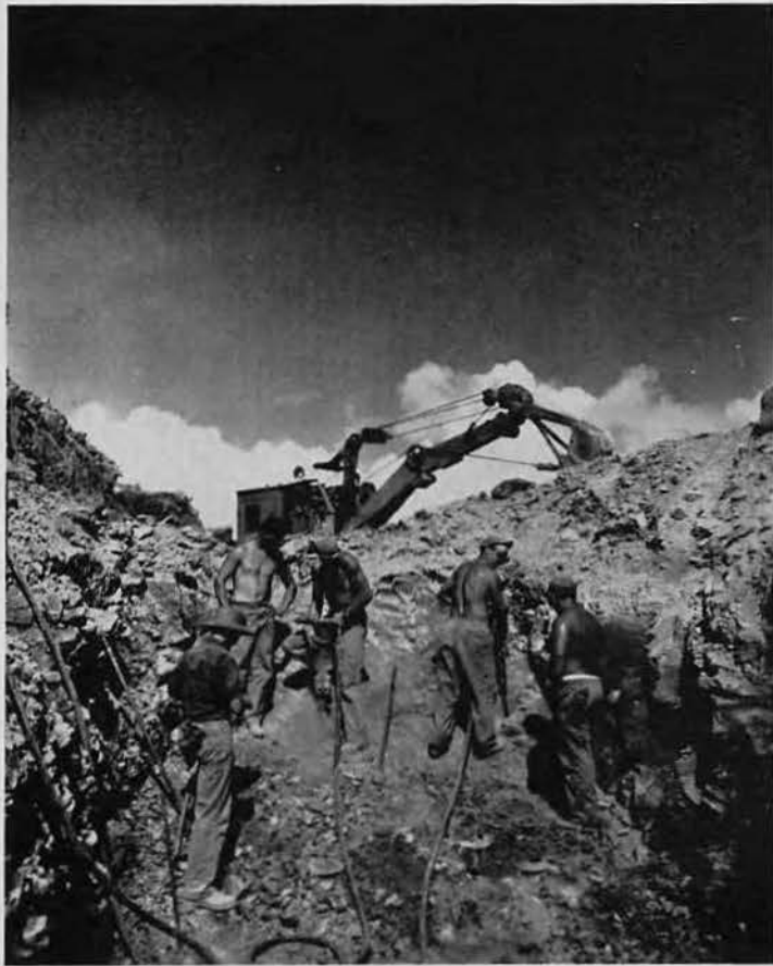
TOUGH SPOT. Preparing to blast stubborn section of shale in center of another drainage ditch, demolition crew is sinking 12-foot holes into rock. Handling chattering jackhammers in intense heat was rugged duty—even for "Mush"!
