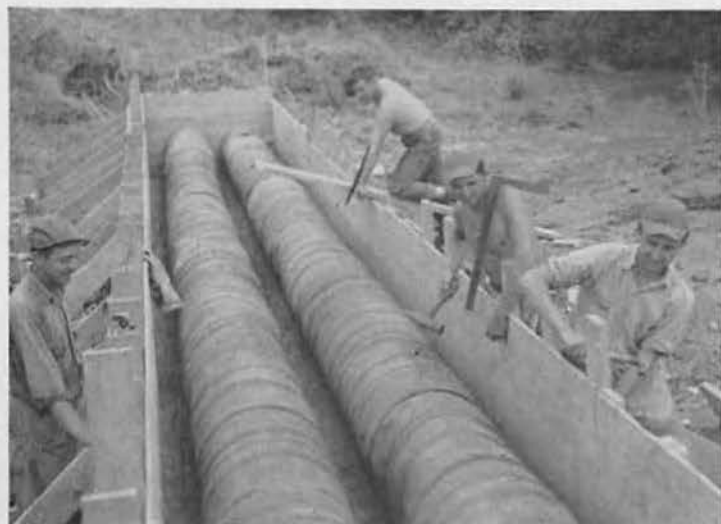
DRUMMERS. Oil drums (with ends out) were spliced together in long double rows and set on concrete foundations for culverts. Carpenters, like Ray Pursley's crew, then built forms around drums for other three sides. Others shown: Nelson, Stuchlik and Straz.
