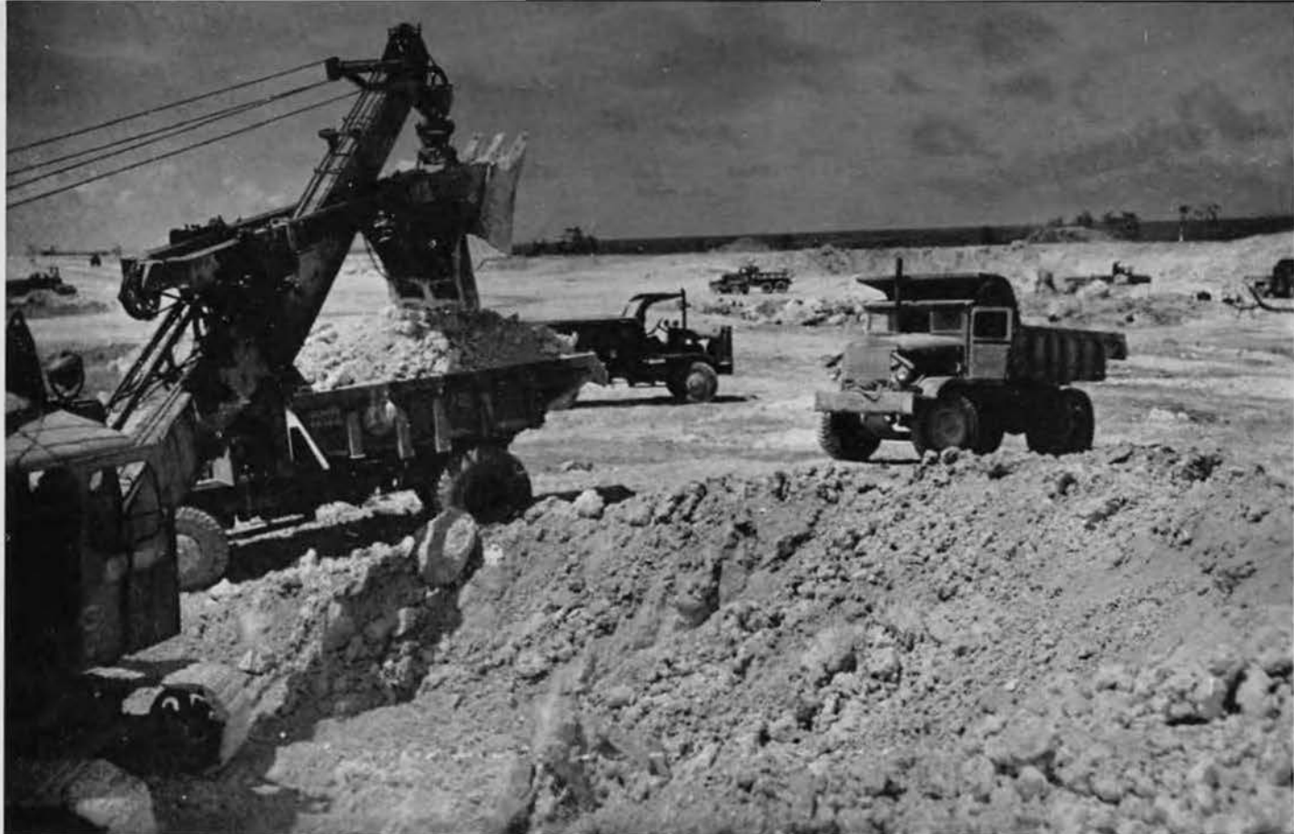
BIG PIT. A 2½-yard shovel and a small fleet of Euclid trucks are working out huge portions of coral at spot known as "the big pit." This site supplied coral for most of runway, plus connecting link with west taxiway.
