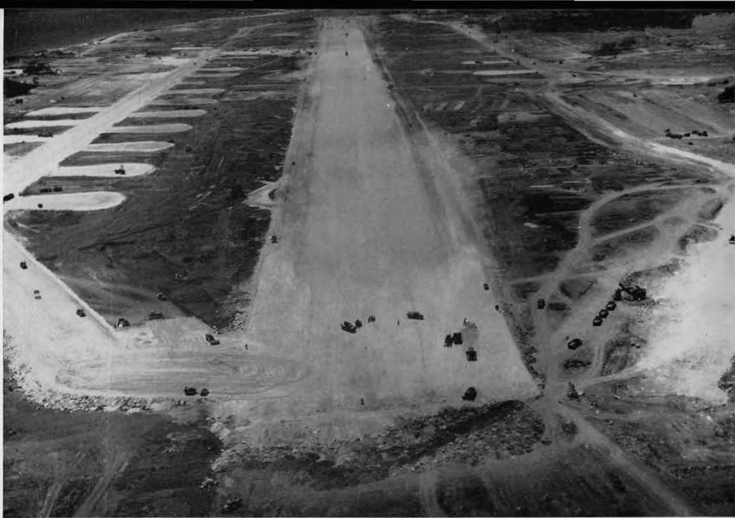
HEAVYWEIGHT! Close-up aerial of Bolo Field, still under construction by 87th Seabees, shows airfield makers and equipment rushing to finish sprawling B-29 strip in time to help deliver knockout blows to hard-pressed Japan. Jackhammer crews remove niggerheads (central fore-
