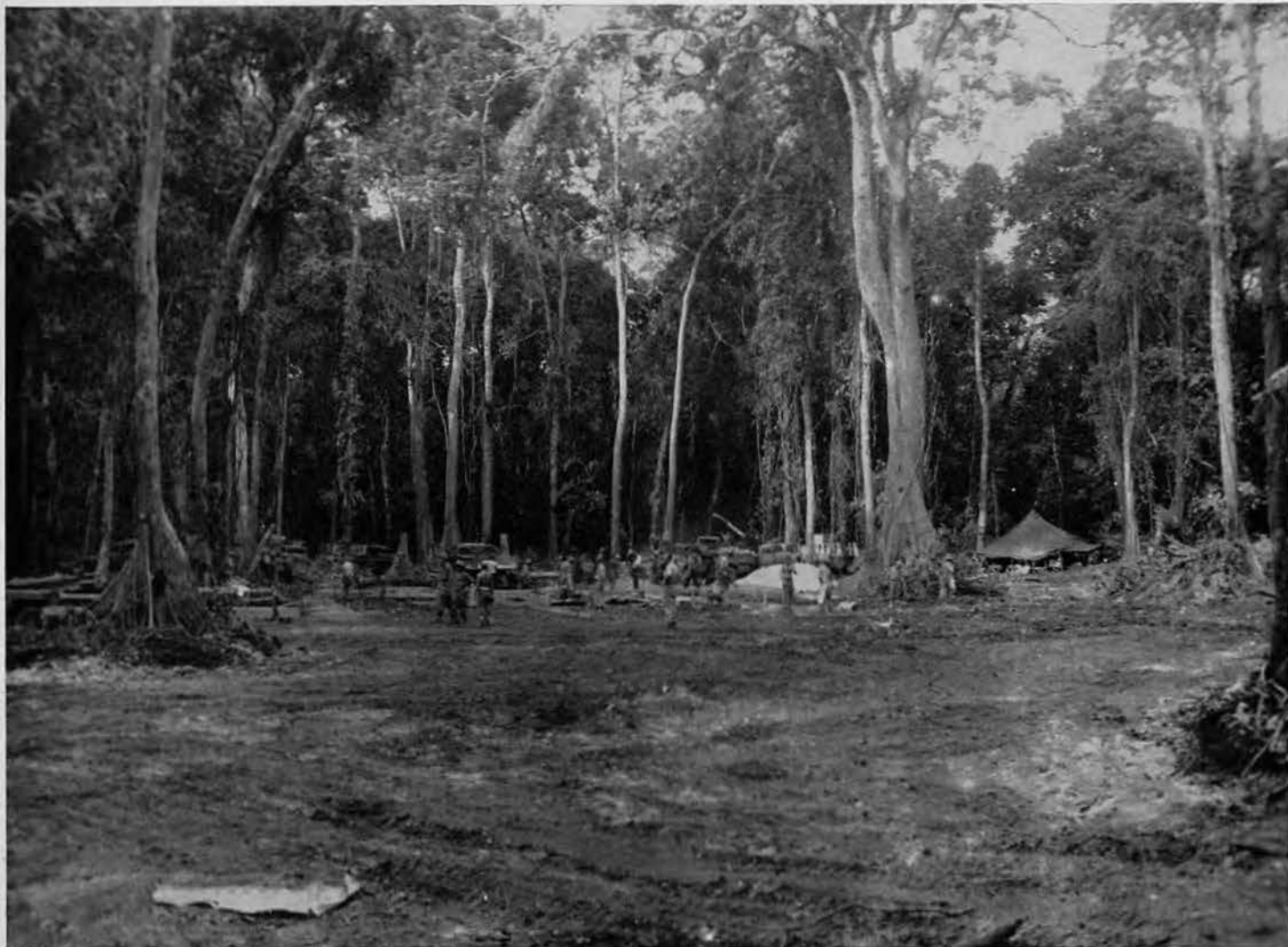
JUNGLE SUFFERS SET-BACK. Not even this almost impenetrable jungle can withstand the Seabees' assault as they labor tirelessly to push back the thick, green mass for the new 87th chow hall. Here, in a neatly bulldozed central clearing, concrete foundations are laid. A hastily-pitched tent
