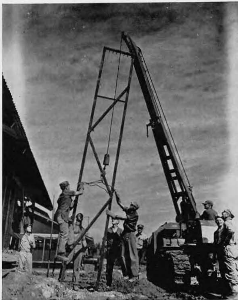
SUPERVISION, PLUS! An officer (Lieut. Davis) and three chiefs (McKinney, Wemple and Rhyne) "supervise" four electricians and crane operator in erecting Jap rails fashioned into light poles for camp area. Workers: Henderson, Scott, Chet Smith, Dobbs. Operator: Carnes.
