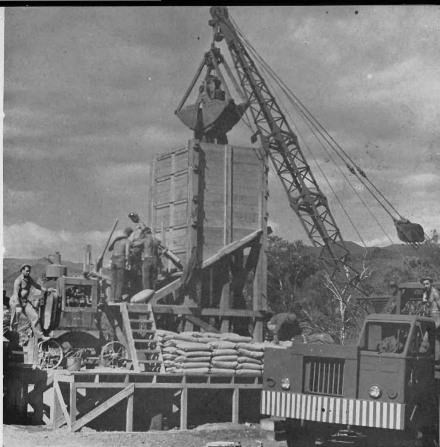
MACHINE AGE. In order to speed the distribution of mixed concrete, a mixing plant was centrally erected in the primary construction area. A clamshell rig was set up next to it. With this convenient arrangement, the aggregate was scraped directly into large, wooden hopper from
