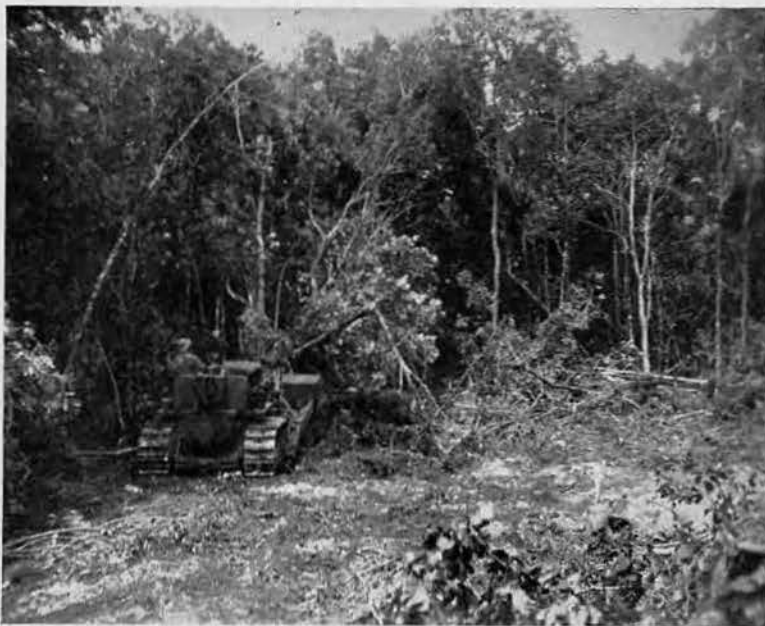
AND THERE WAS LIGHT. The jungle begins to recede from the onslaughts of the big 'dozers. Things are looking better as the boys break into their theme song, "Move It Over." (This picture appears on Page LX of CAN DO, "The Story of the Seabees.")
