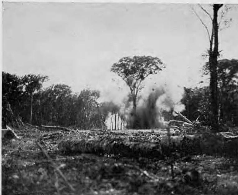
BLOWING IT OUT. Stalwarts like this required a little extra persuasion. This 48-incher, which is held up by large buttressing roots, proved too difficult for the 'dozers. A little "Can Do" and a shot of dynamite finally did the trick.
