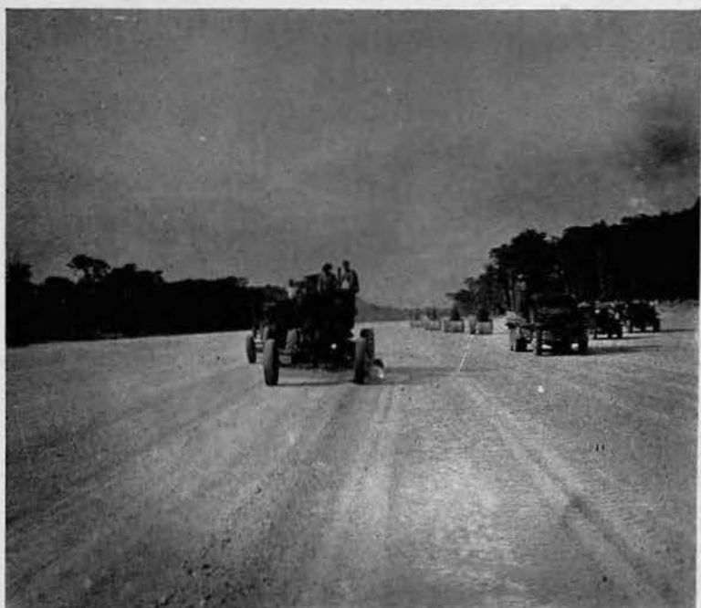
PERFECT FORMATION. Tandem lines of graders and rollers are shown during "face-lifting" operation performed on Stirling Field runway early in June. Harvil Nolin and George Sambrat, equipment operators, are leading grader parade. Work was continuous for two days and nights.
