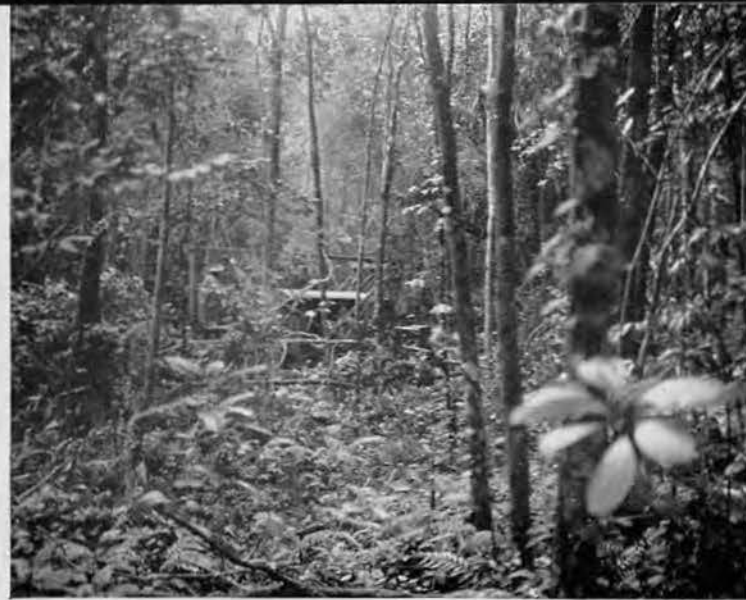
LET THERE BE LIGHT! This isn't a night clearing scene. It was just this dark when the first bulldozer arrived on the centerline of Stirling Strip the first morning of clearing operations. Lights were soon installed in the virgin jungle.
