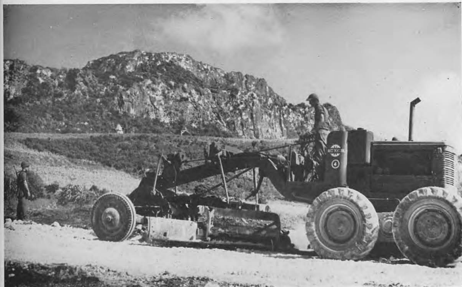
JOB VARIETY. A guard stands solitary watch as John Bell guides motor grader over rough coral road within staging camp perimeter. Dazzling coral surface gave off constant clouds of powdery dust and men and tents became coated with grimy skim of dirt. De-
