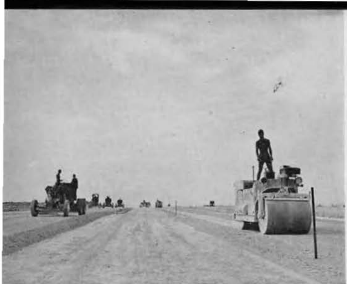
ON THE BALL. Grader and roller operators exert best effort to get everything in readiness for the final paving as Superforts are soon due. William Young (on roller) stands for better view as machine comes near a grade stake.
