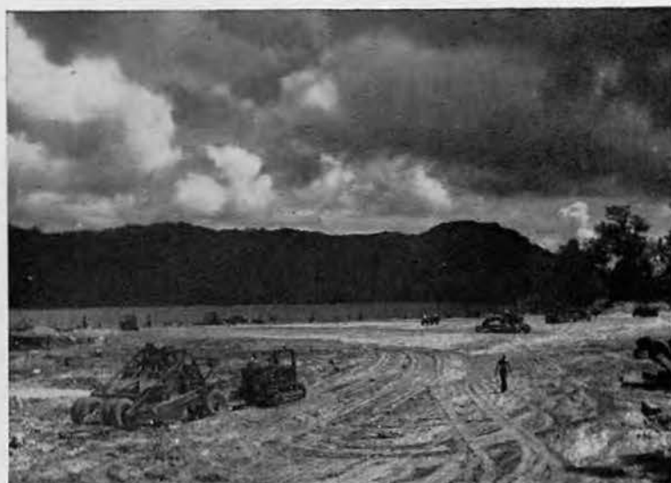
HILL DISAPPEARS. Grading of the cleared dock area is now progressing by leaps and bounds. The hill, which formerly was here, has been carved away and used as fill on shore access road. Plane tender is anchored offshore with PBYS.
