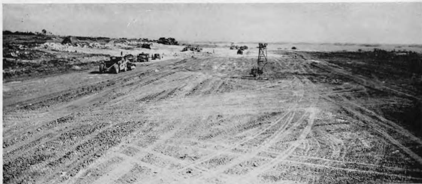
SOUTH END of runway begins to take on a semblance of grade completion after a sustained siege of clearing, cutting and filling. Coral (left center) came from huge drainage cut and was spread by pans as prelude to heavy laying of coral by trucks. Light towers (center) provide
