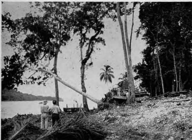
POWER. Initial clearing for Stirling Dock area begins. Jack Kenning (on D-8) pushes over sizeable tree—roots and all, thereby providing more fodder for the battalion sawmill. A stubby LCM plys its route between Stirling and Mono.
