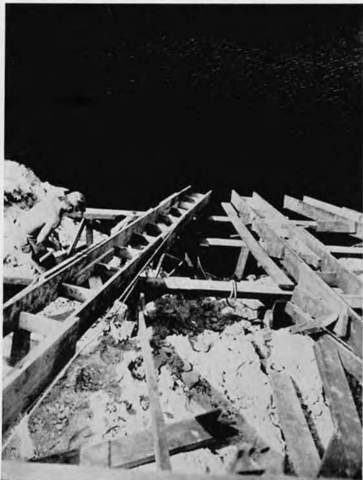
IT'S A LONG WAY DOWN, but Stacy Potter, member of a carpenter crew building foundations for three oil drum chutes designed to carry garbage 75 feet down to the sea, keeps right on with his tedious form work. (For view of completed chutes, see picture above.)
