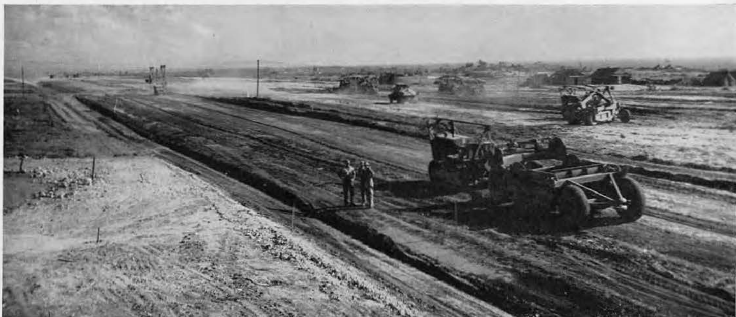
STRAIGHT AWAY. Invaluable pans are seen grading just east of coral hill shown above. Through clouds of dust (left), fast rolling trucks may be seen dumping loads of coral at start of runway. Some buildings and tents of the Seventh Marine Field Depot are still here (left and right),
