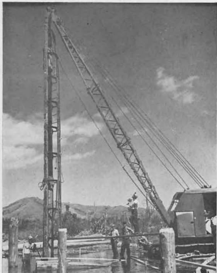
MILES OF PILES. Battalion pile-driver assembly more than earned its keep. Shuttling from one bridge to another, the Northwest "25" rig, with its 2,000-pound hammer, kept ramming the long piles into the earth until last day of construction.
