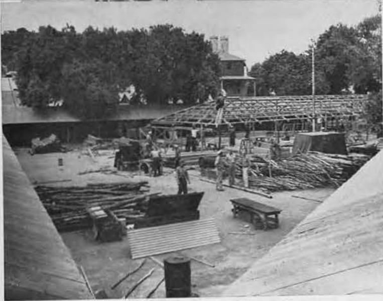
GOOD START. Carpenter crews of Chiefs Emil Schoenke and Frank Lutterall were assigned the construction of a servicemen's center in the heart of Noumea. A concrete deck (easy to clean with hose and water) has hardened as building commences.
