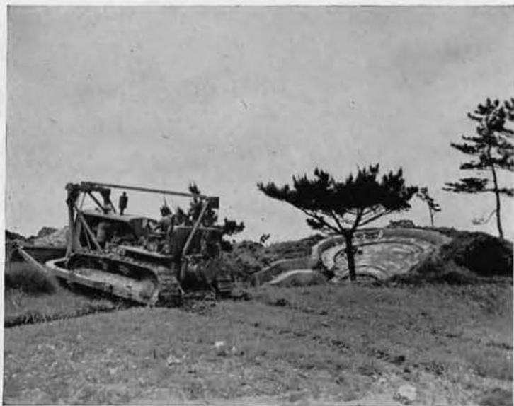
DO NOT DISTURB. Cliff Engebretson comes dangerously close to disturbing the peace of native ancestors as he breaks the solitude by leveling a revetment for a gasoline dump. These nicely designed tombs were found just about everywhere on Okinawa.
