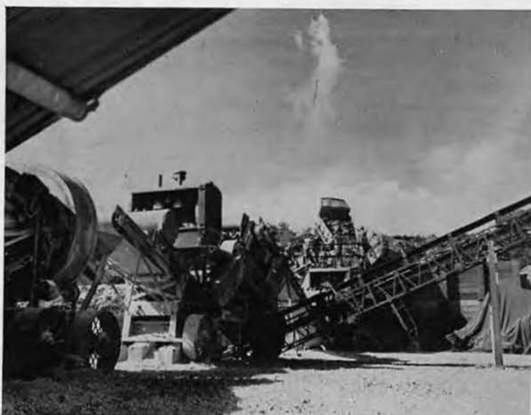
THE WORKS. Here is an overall view of entire unit in operation from time rough rock is dumped into crusher (center) until it is carried up conveyor belts ready for use. Nearby quarry was considered a dangerous assignment.
