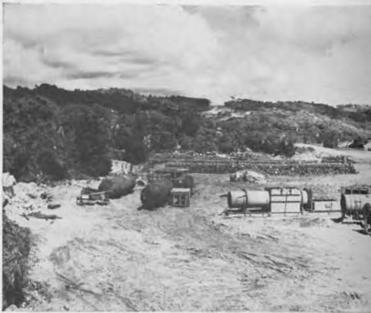
ASPHALT PLANT. The 87th's ability to absorb punishment (and endless work assignments!) was again demonstrated when the battalion fell heir to the new asphalt plant set up at Nagahama. However, it soon went to 82nd Seabees.
