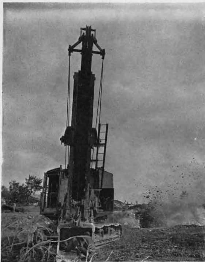
TAKE COVER! Shovel operator and his oiler curl up inside huge dipper (left foreground) as demolition crew shoots out a tough baby in center of runway. Heavy steel of bucket provides ample protection against flying debris.
