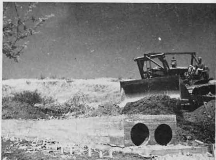
OVER THE TOP! Once the concrete had sufficiently hardened, wooden forms were stripped off and the indispensable bulldozers bladed tons of earth over the drains to bring spot to road level. Grady Thompson (at controls) shows how it's done.
