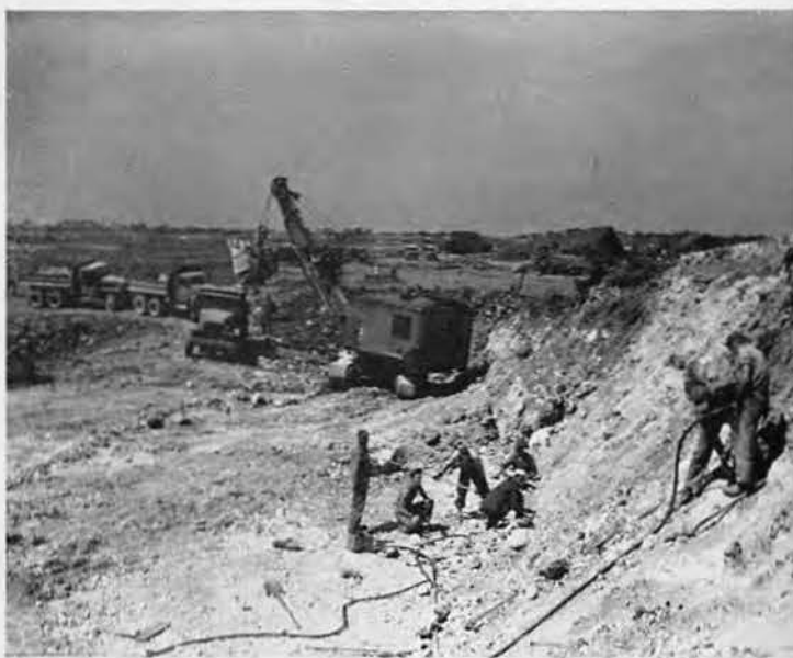
GRAND OPENING. A power-shovel starts cutting into one of the two coral pits that are to provide all paving material for the Bolo job. Demolition gang drills hole for charge to loosen up solid portions of the coral formation.
