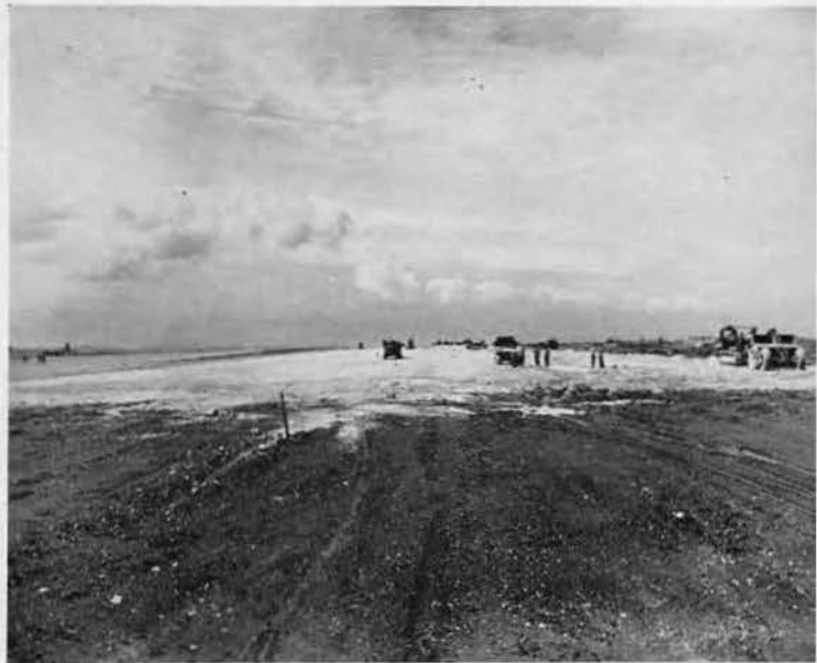
CONSTANT RAINS have turned sub-grade into a bog. Pans have been brought back to work over the wet coral. All finishing work is practically at a standstill, but the gang is loading chunks of rock removed from surface to utilize time.
